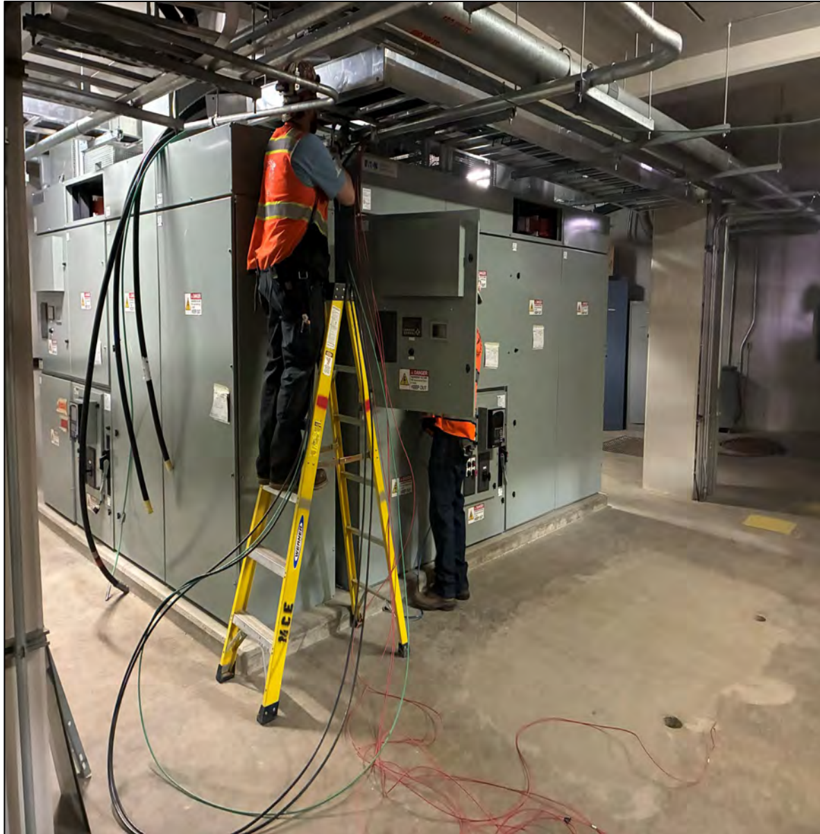
Figure 3 – Control Cable Pull from Level B1 to Level B2 Gear @ Chapaton PS
