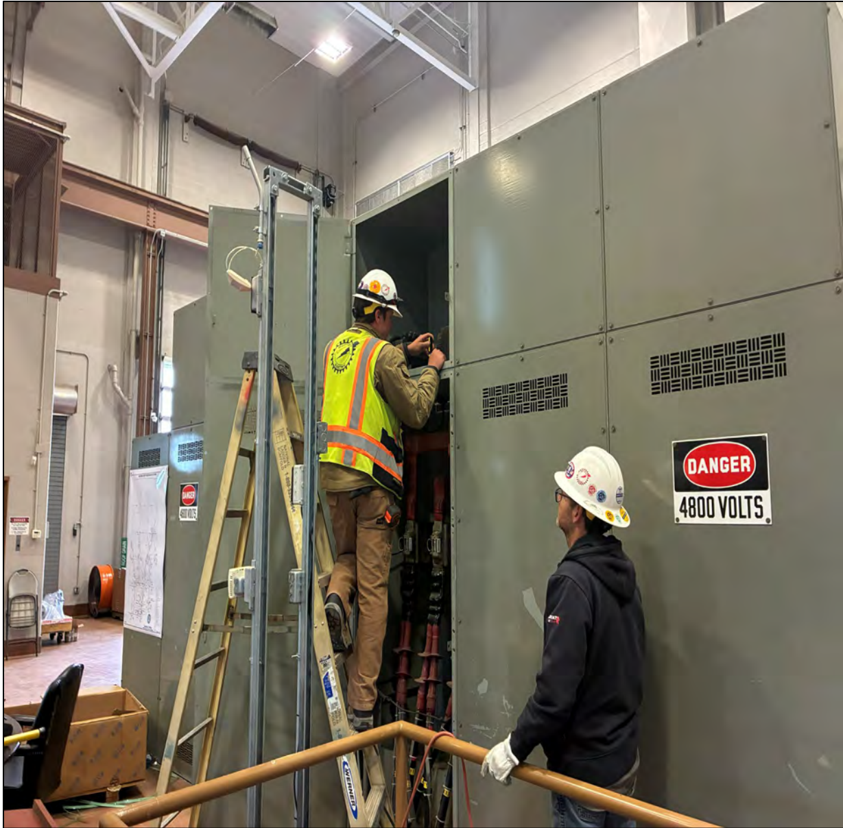
Figure 4 – Existing Gear Connection Check for DTE Splice @ Chapaton PS
