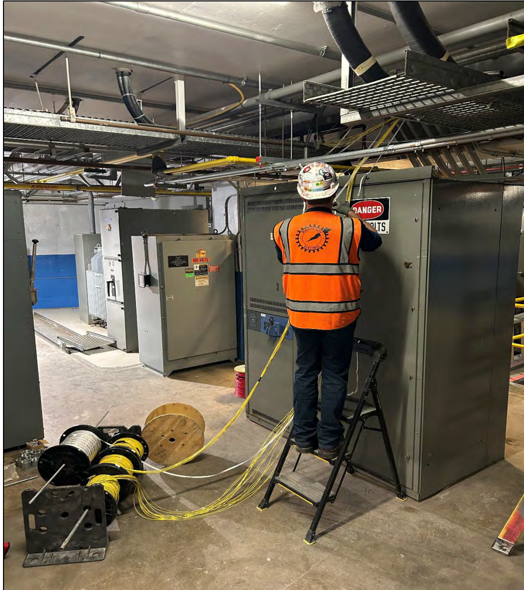
Figure 2 – Control Cable Pull from Main Floor Level thru Level B1 @ Chapaton PS
