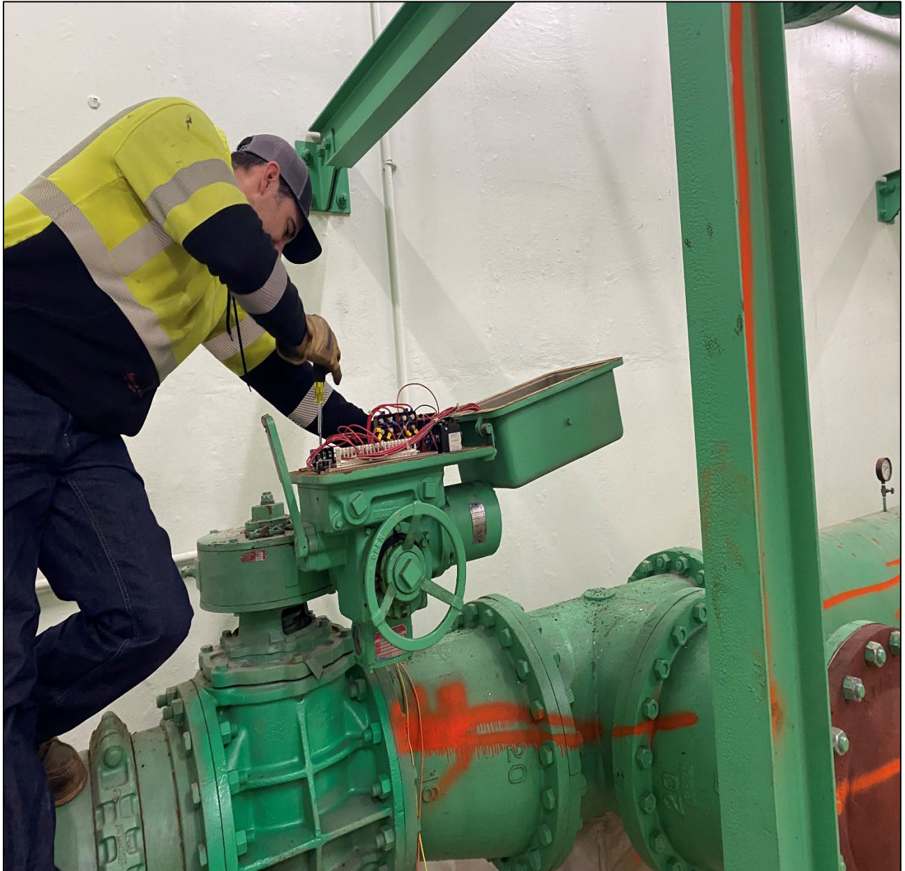
Figure 1 –Electrician Disconnecting Electrical Martin RTB Pipe Gallery
