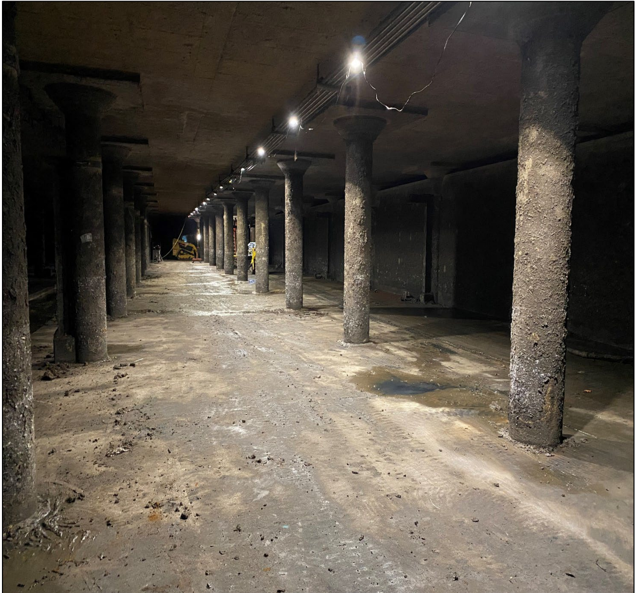
Figure 7 – Temporary Work Lighting in Martin RTB
