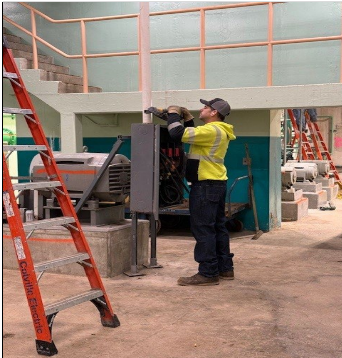
Figure 2 – Electrician Disconnecting Electrical Martin RTB Pipe Gallery
