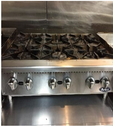
Counter top equipment elevated on 4-inch legs to provide space for cleaning underneath
