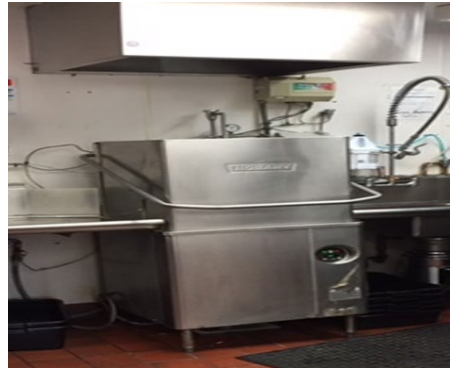
Type II hood over heat/moisture producing dishmachine
