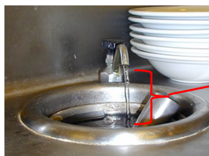
Air gap between water supply line and flood rim of receptacle
