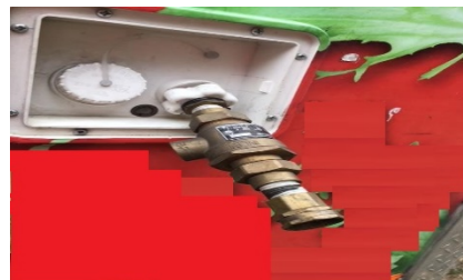
Backflow preventer installed on exterior of unit for connection of public water line
