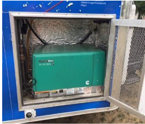
Generator installed in exterior compartment of unit
