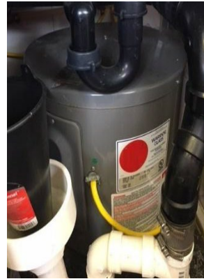
Tank water heater
