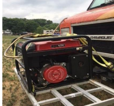
Generator installed outside of unit
