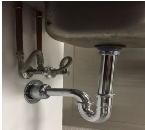
Direct connection- not permitted on equipment in which food, portable equipment or utensils are placed
