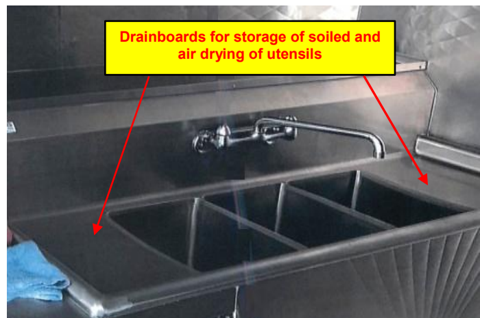
Fixed 3-compartment set up with drainboards
