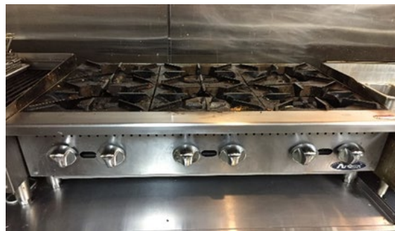
Equipment Elevated 4" Above Counter
