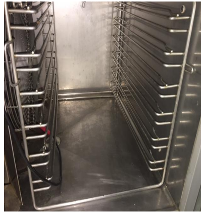
Interior of Blast Chiller
