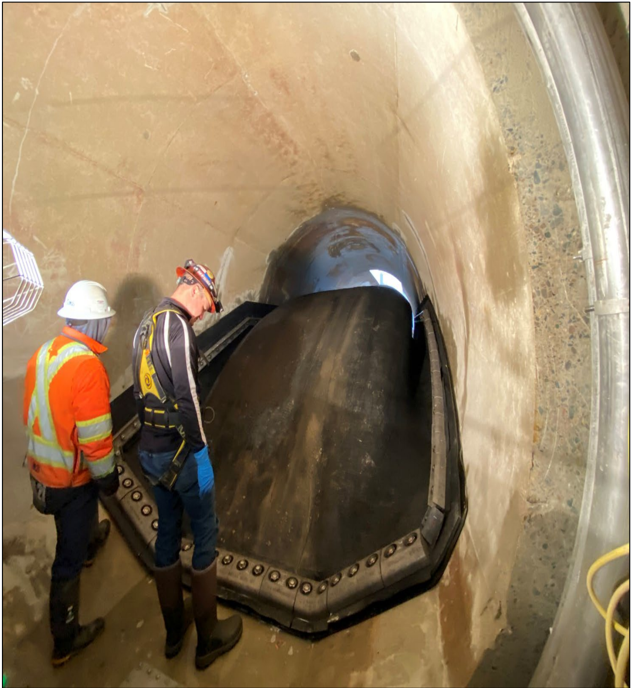
Figure 12 – Inflating Sewer Gate @ 11.5FT Tunnel
