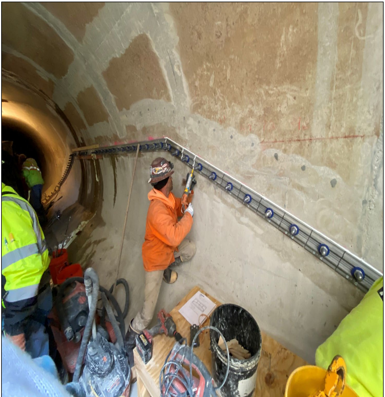
Figure 7 – Anchors and Inflatable Dam Mounting Plates @ Beaconsfield 11.5 FT Tunnel
