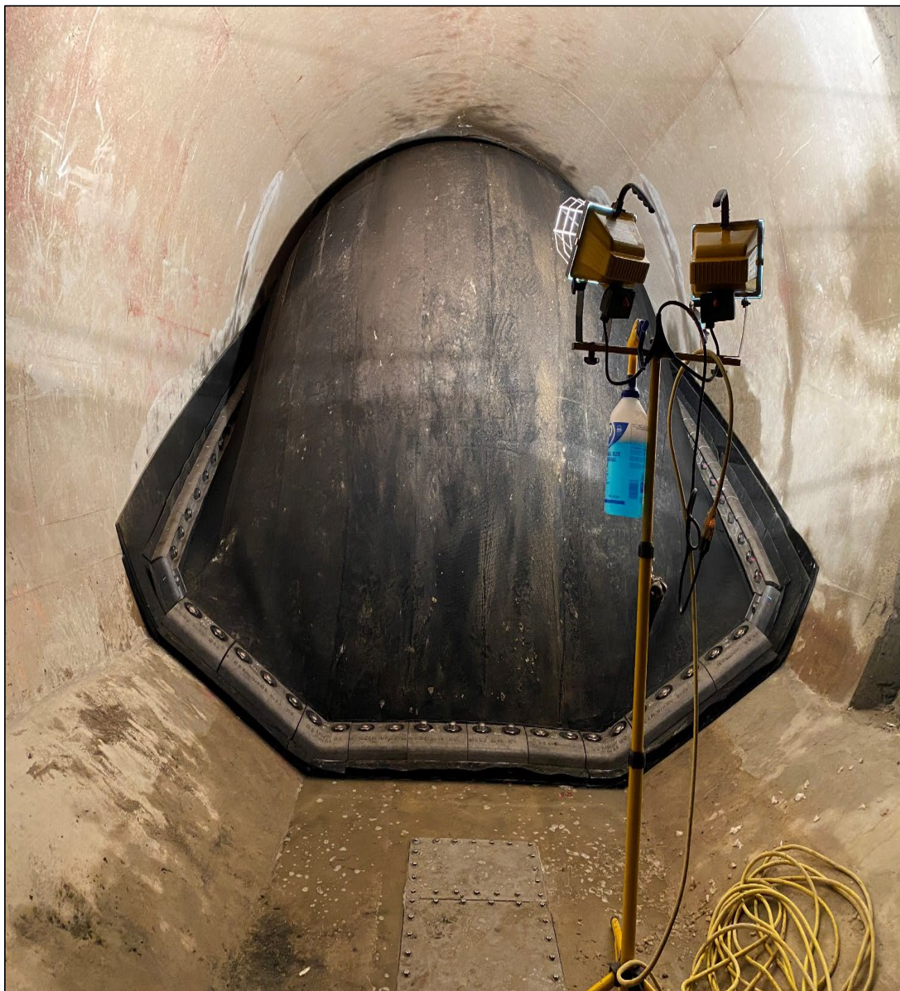
Figure 13 –Inflated Sewer Gate to Crown of Pipe @ 11.5FT Tunnel
