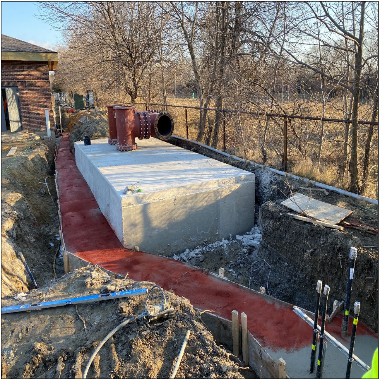
Figure 2 – Concrete Elect. Duct Bank w/Red Dye @ Beaconsfield Rd.
