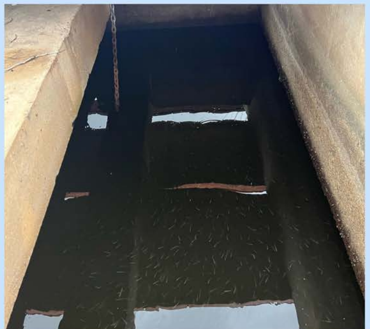
Minnows seen in the trash capture structure two weeks after litter was removed.
