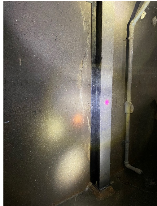
Figure 6 – Concrete delamination at flushing pipe support
