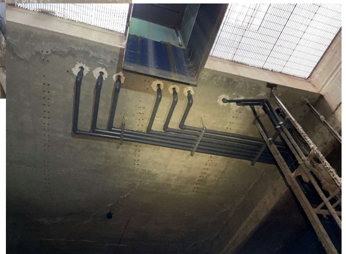
Figure 3 – New 2" sample piping through floor into Blower Room
