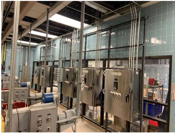
Figure 1 – Five new VFD cabinets to power Hose Pumps
