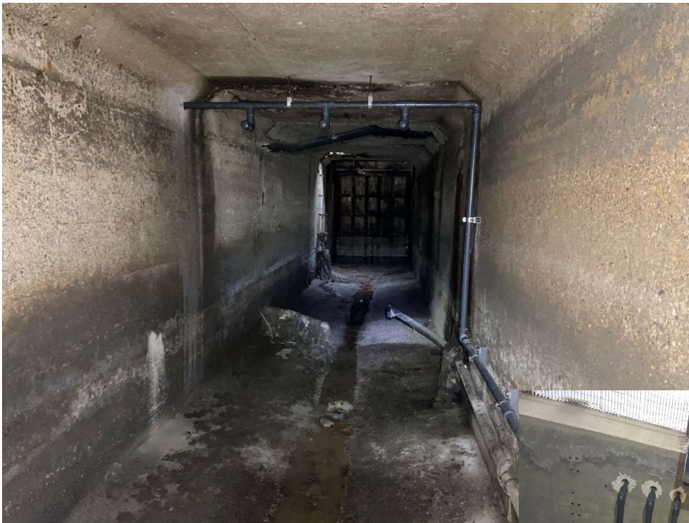
Figure 2 – New 9-Mile Box Chlorine Diffuser – North box, just east of Tide Gates
