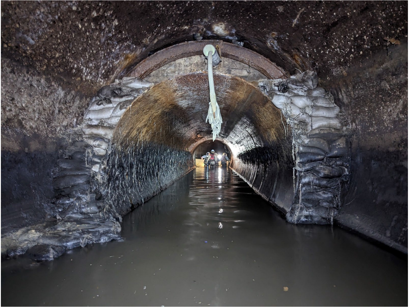
Figure 7 – Verifying Dimensions for Partial Height Bulkhead near CS-12 to facilitate removal of the temporary flume
