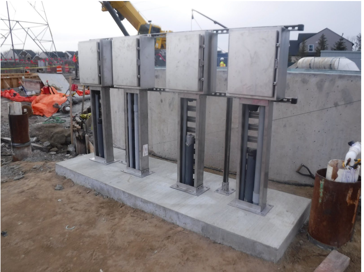
Figure 6 – CS-12 Electrical Termination Boxes for Pumps
