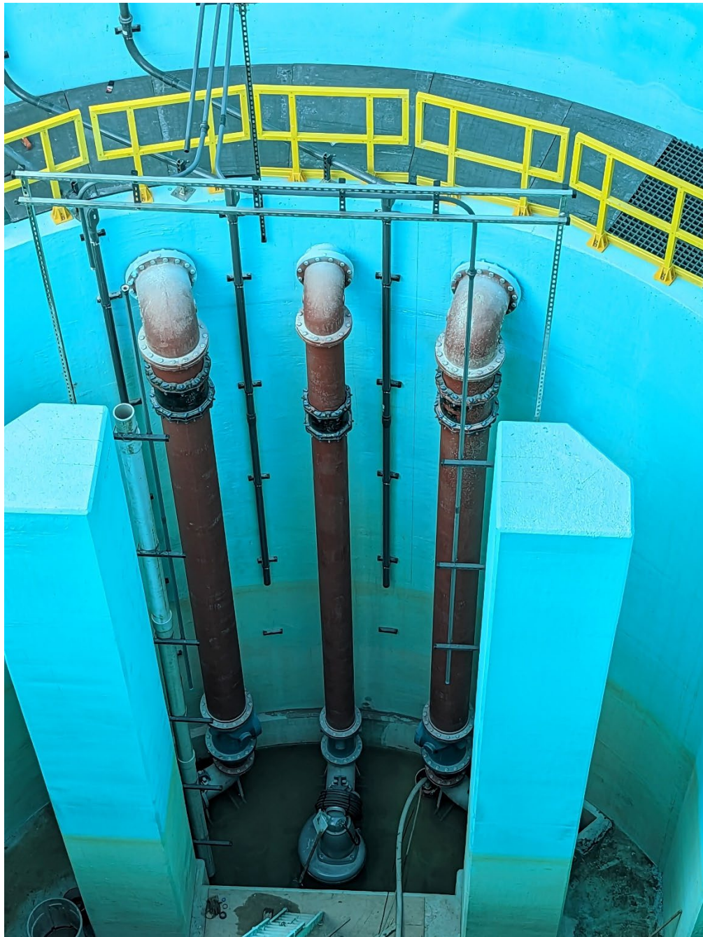
Figure 2 - CS-12 Pumps – East Side of Structure
