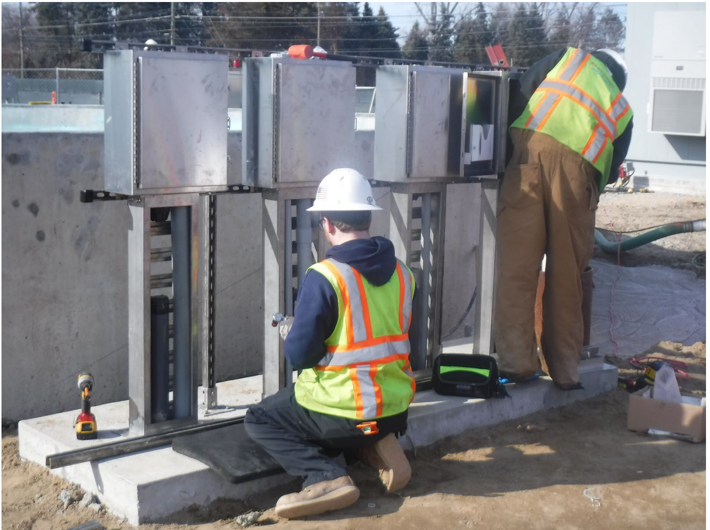
Figure 5 - CS-12 Electrical Termination Boxes for Pumps (east side)
