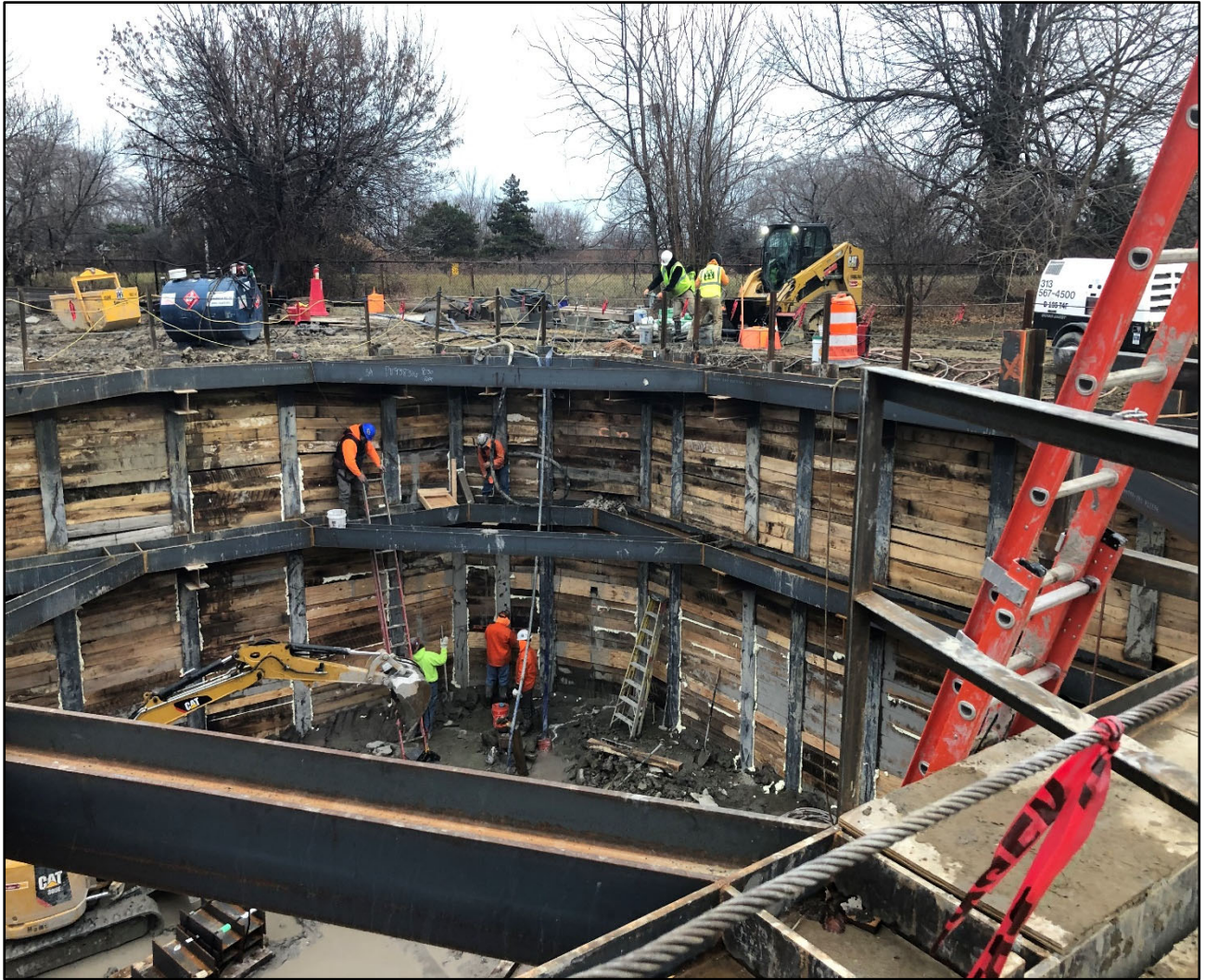
Figure 1 – Grouting Voids Behind Timber Retaining Wall
