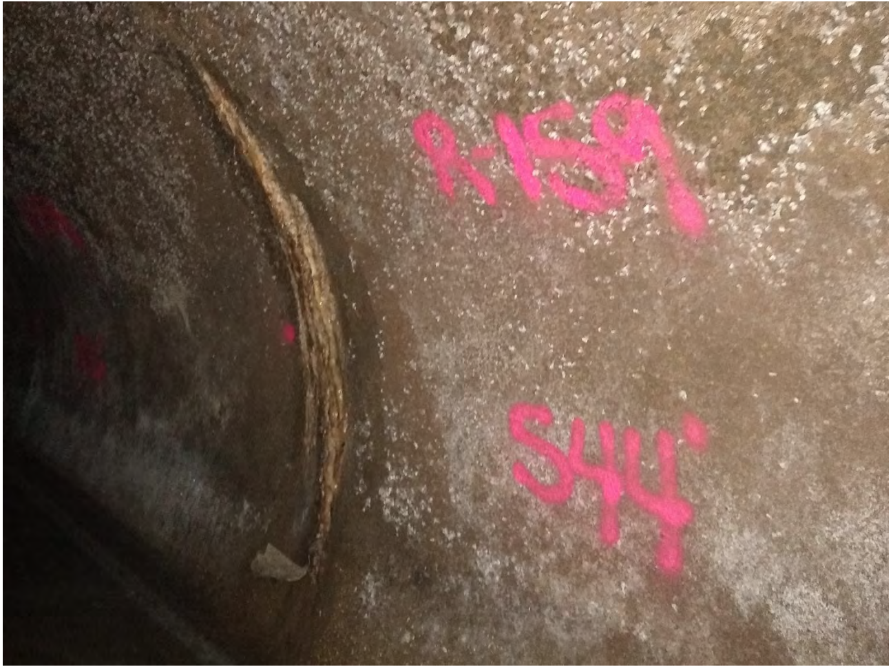
Figure 7 - Typical Infiltration Near MH-019
