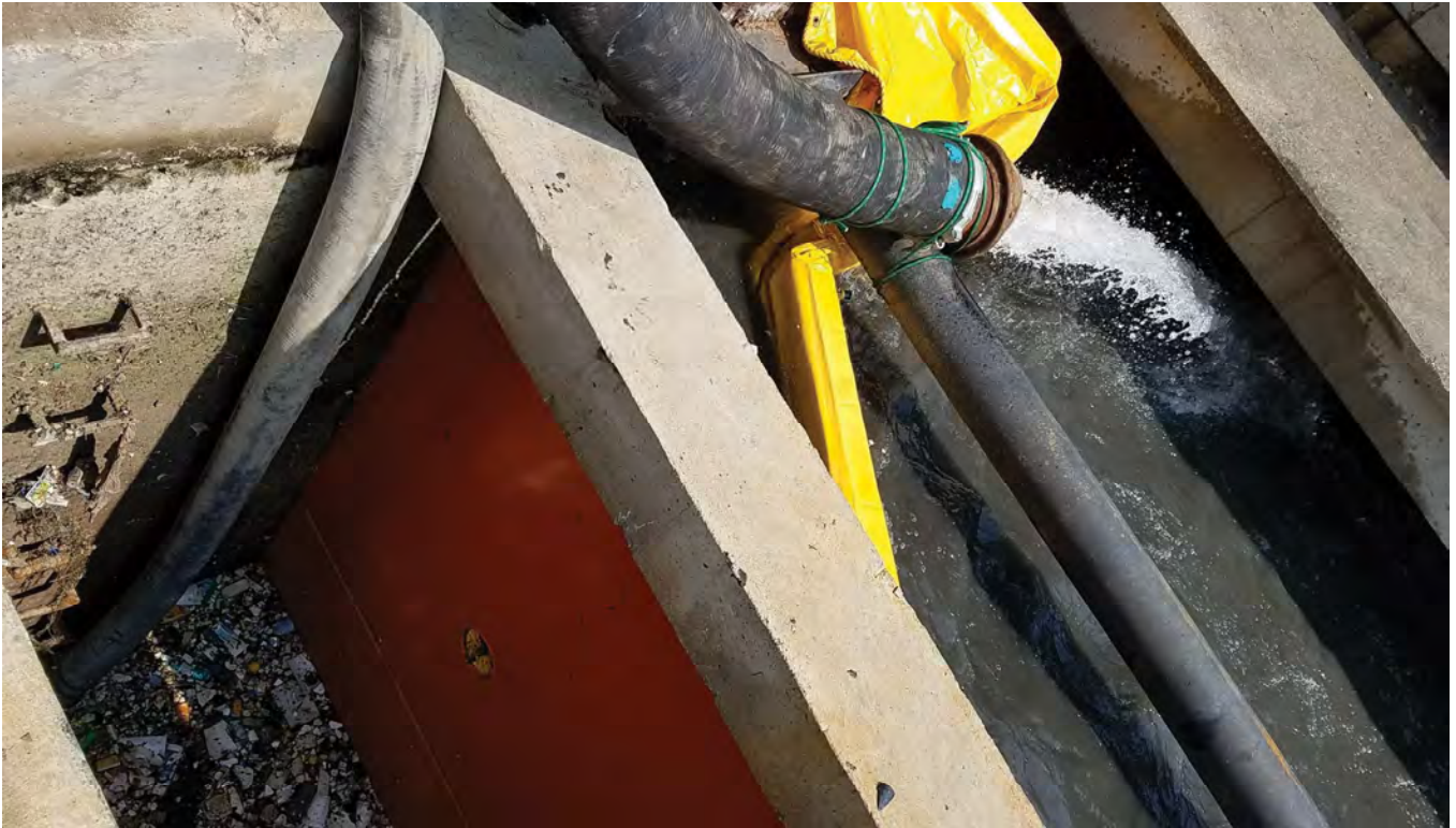
Trash and debris observed during 2018 dewatering
