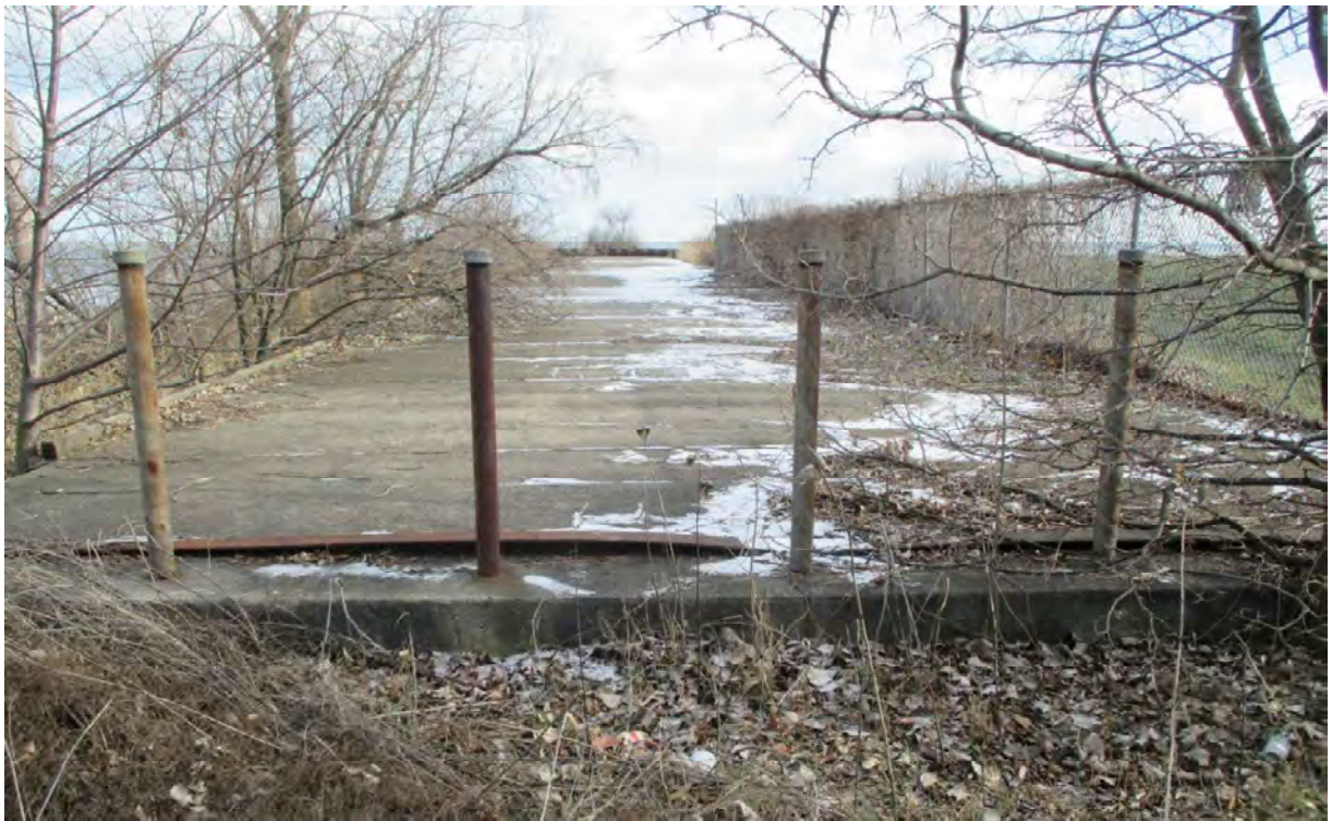
End of pipe and bulkhead with concrete decking looking towards Lake St. Clair
