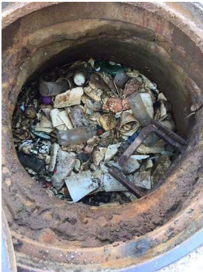
Floatable trash collecting at Jefferson Avenue manhole
