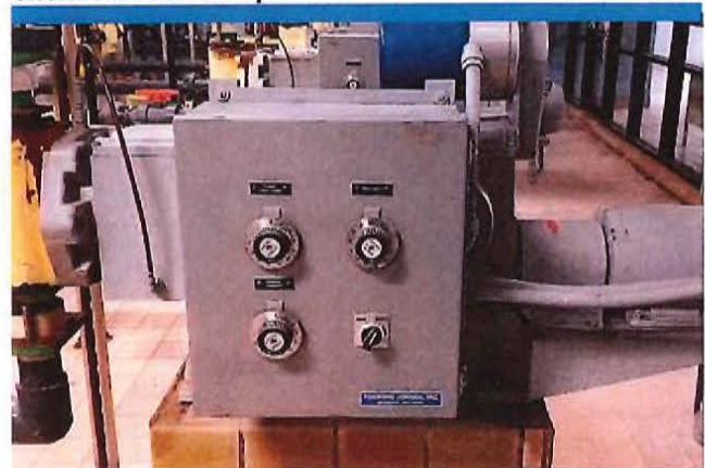
The chemical feed pumps at both Chapaton and Martin Basins require upgrading because replacement parts are no longer available from suppliers.
