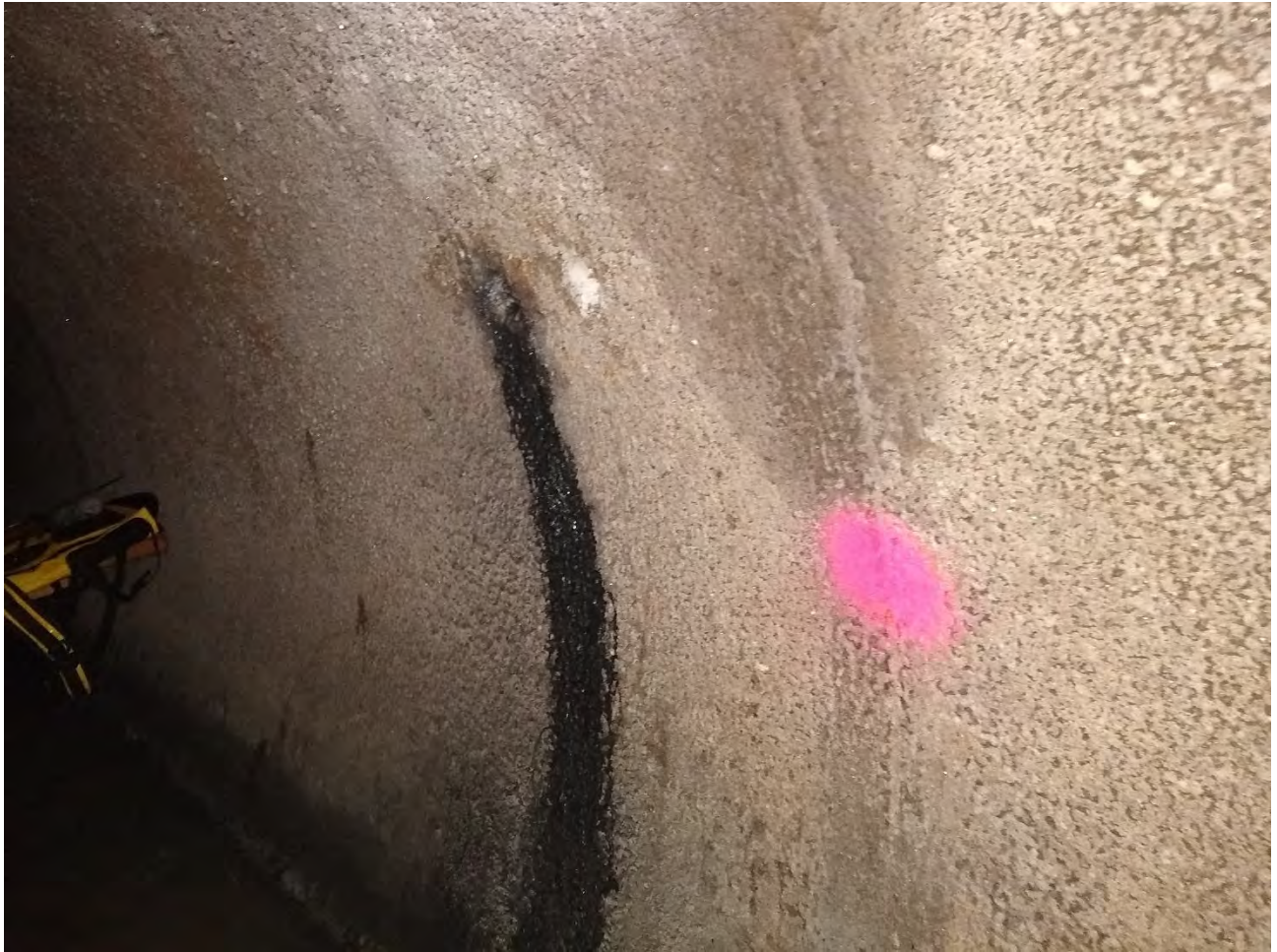
Figure 8 - Typical Infiltration in this Area
