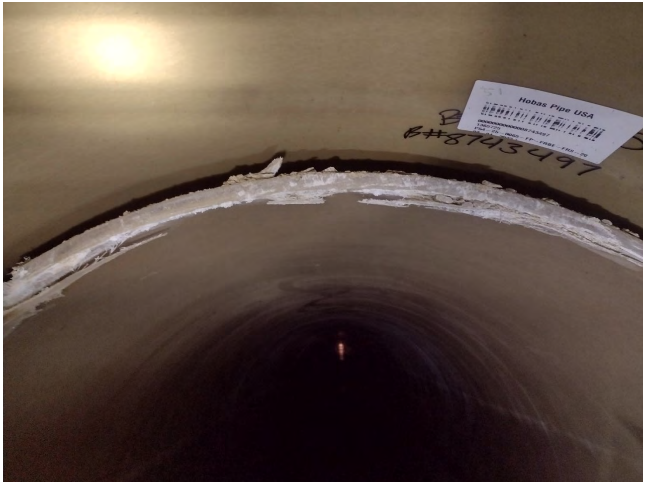
Figure 15 - Severely Damaged HOBAS Joint
