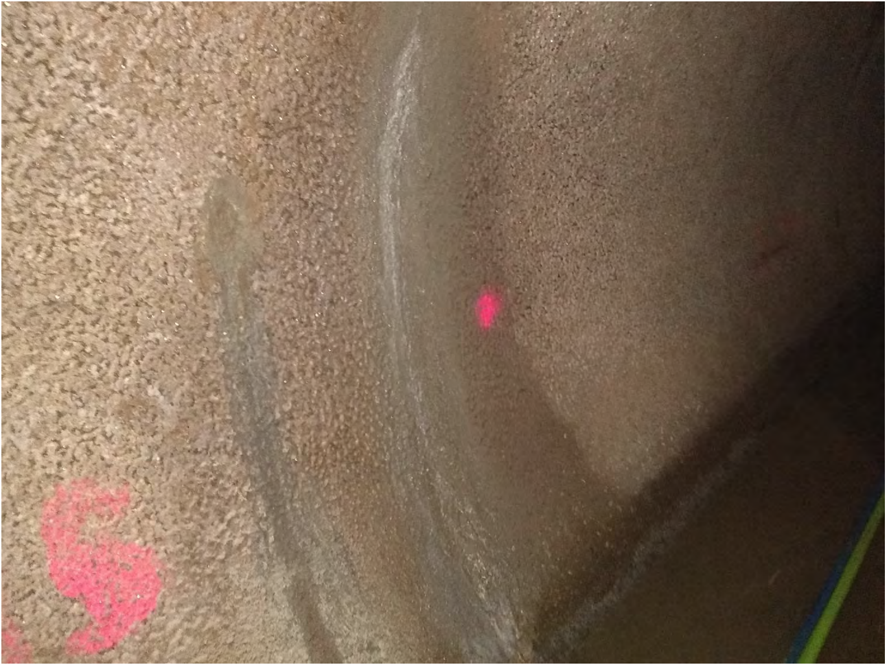
Figure 9 - Typical Infiltration in this Area
