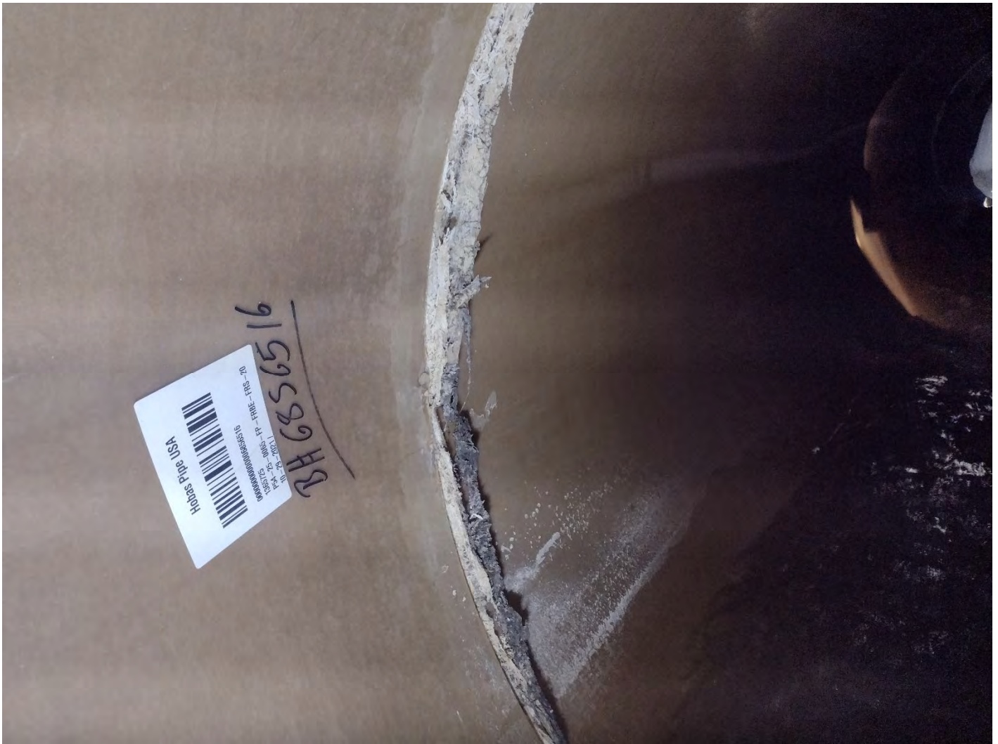
Figure 13 – Damaged HOBAS Joint
