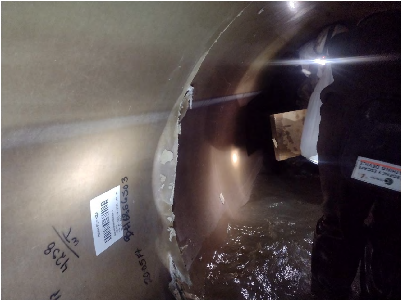
Figure 14 - Damaged HOBAS Joint
