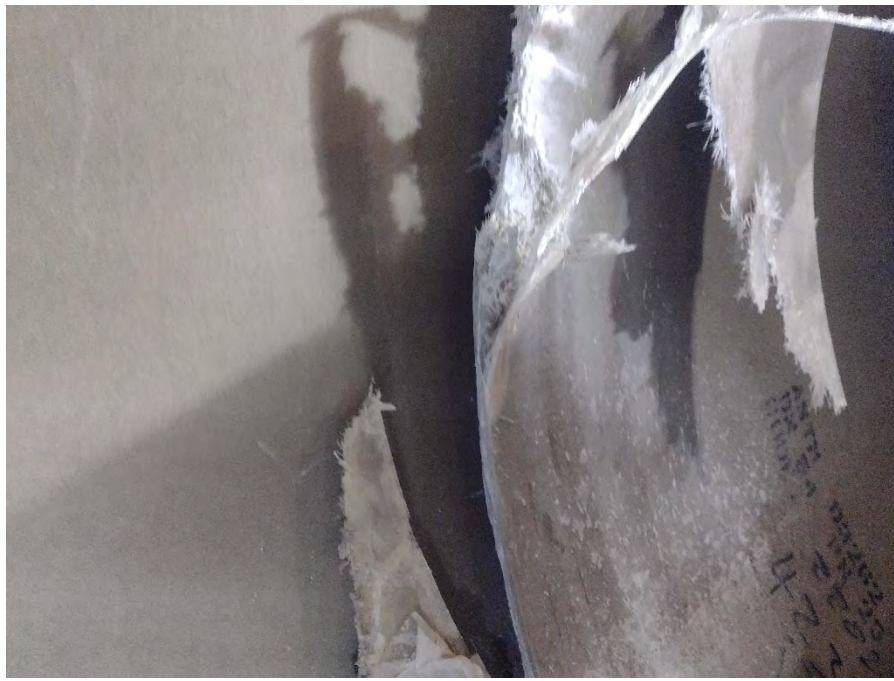
Figure 16 - Severely Damaged HOBAS Joint
