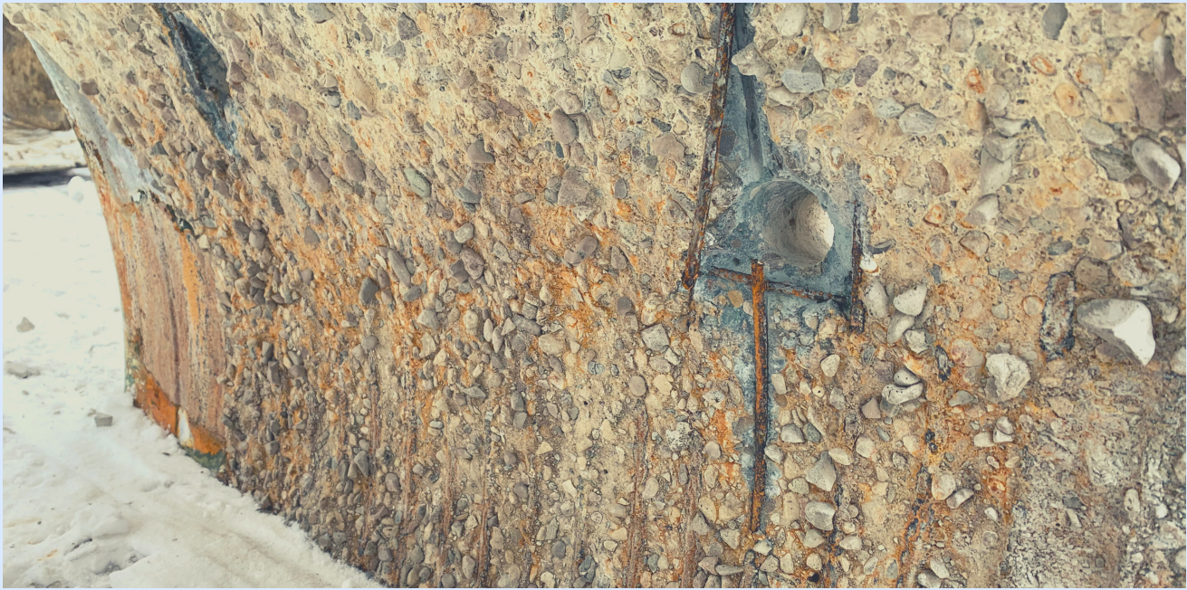
Degradation shown of removed pipe at Segment 6
