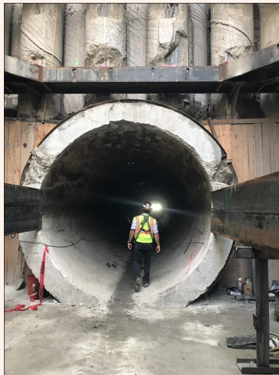
The view into the MIDD Interceptor during the repair process, early August.
