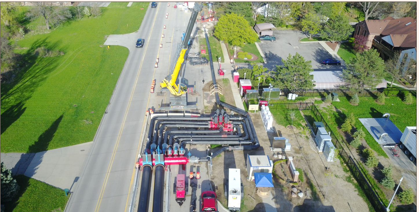
The pump system created to lift sewage from 60 feet below grade and by-pass collapsed portion of the interceptor, April 2017.
