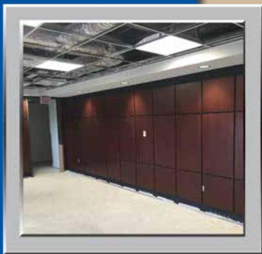
Wood panels are installed in the Friend of the Court hearing rooms.
