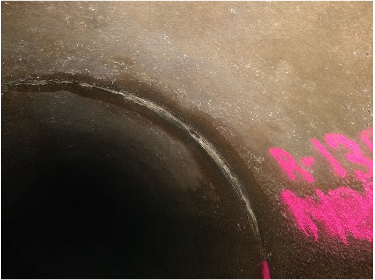
Figure 7 - Typical Infiltration Near MH-19
