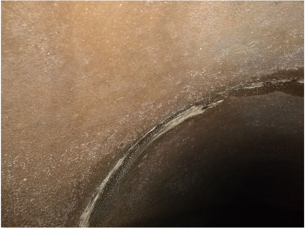
Figure 6 - Typical Infiltration Near MH-019
