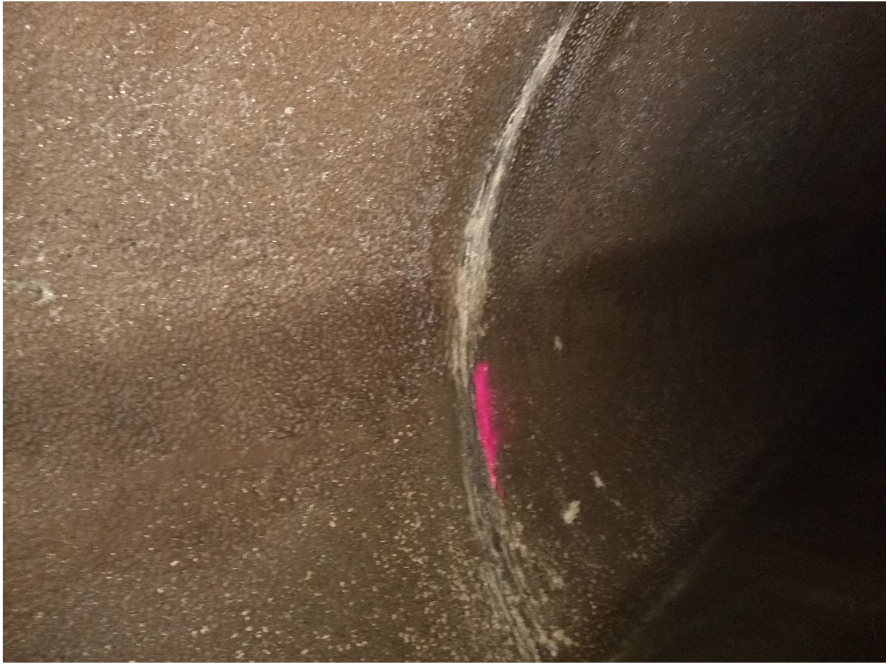
Figure 5 - Typical Infiltration Near MH-19
