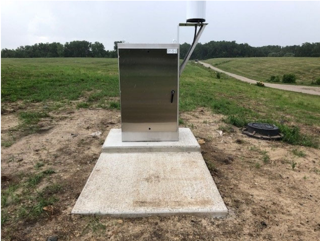
Figure 7 - New Electrical Cabinet at SY-S-2
