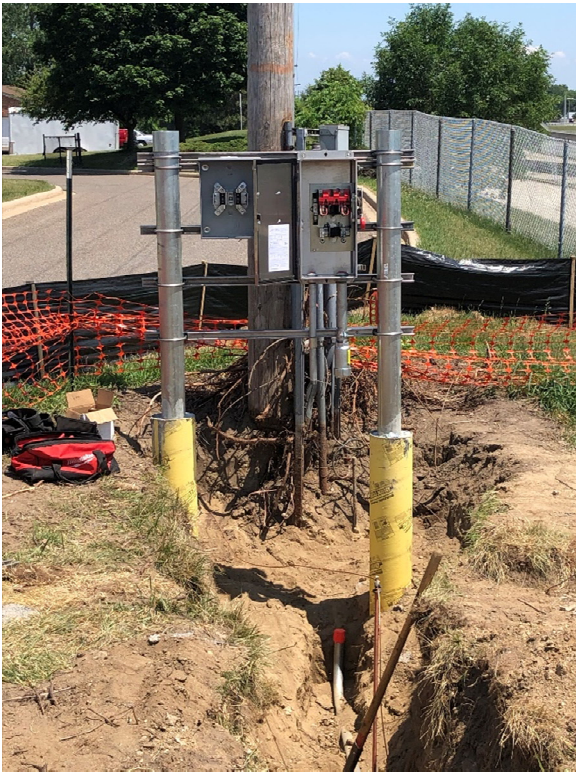
Figure 10 - New Electrical Rack at SY-S-1
