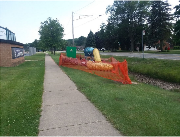
Figure 7 - Ventilation Set-up Near I-94
