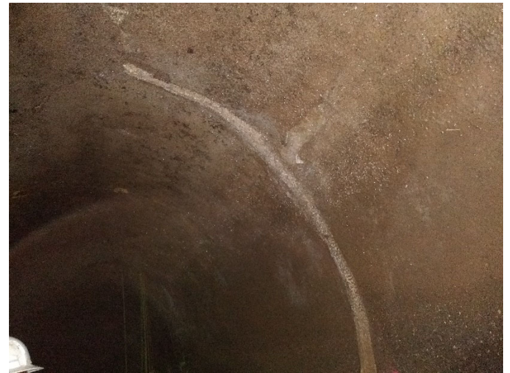
Figure 4 - Infiltration at Crown of Interceptor
