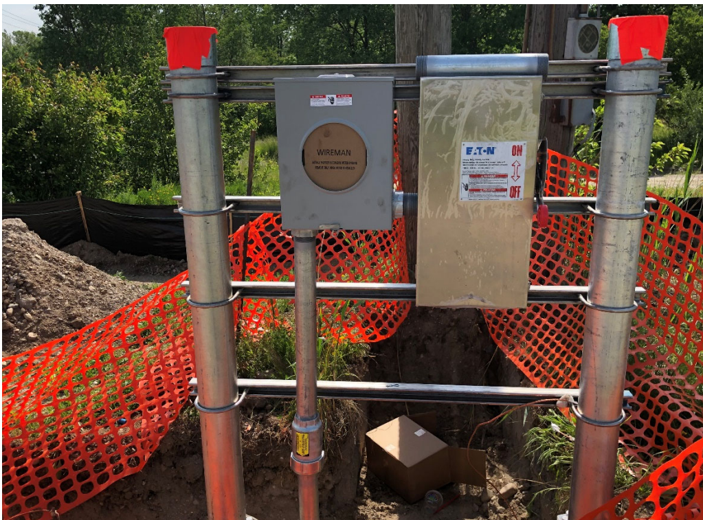
Figure 13 - New Electrical Rack at SY-S-2
