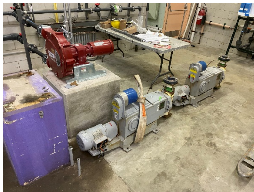
Figure 1 – Old Pulsafeeder disinfection pumps (1978)
