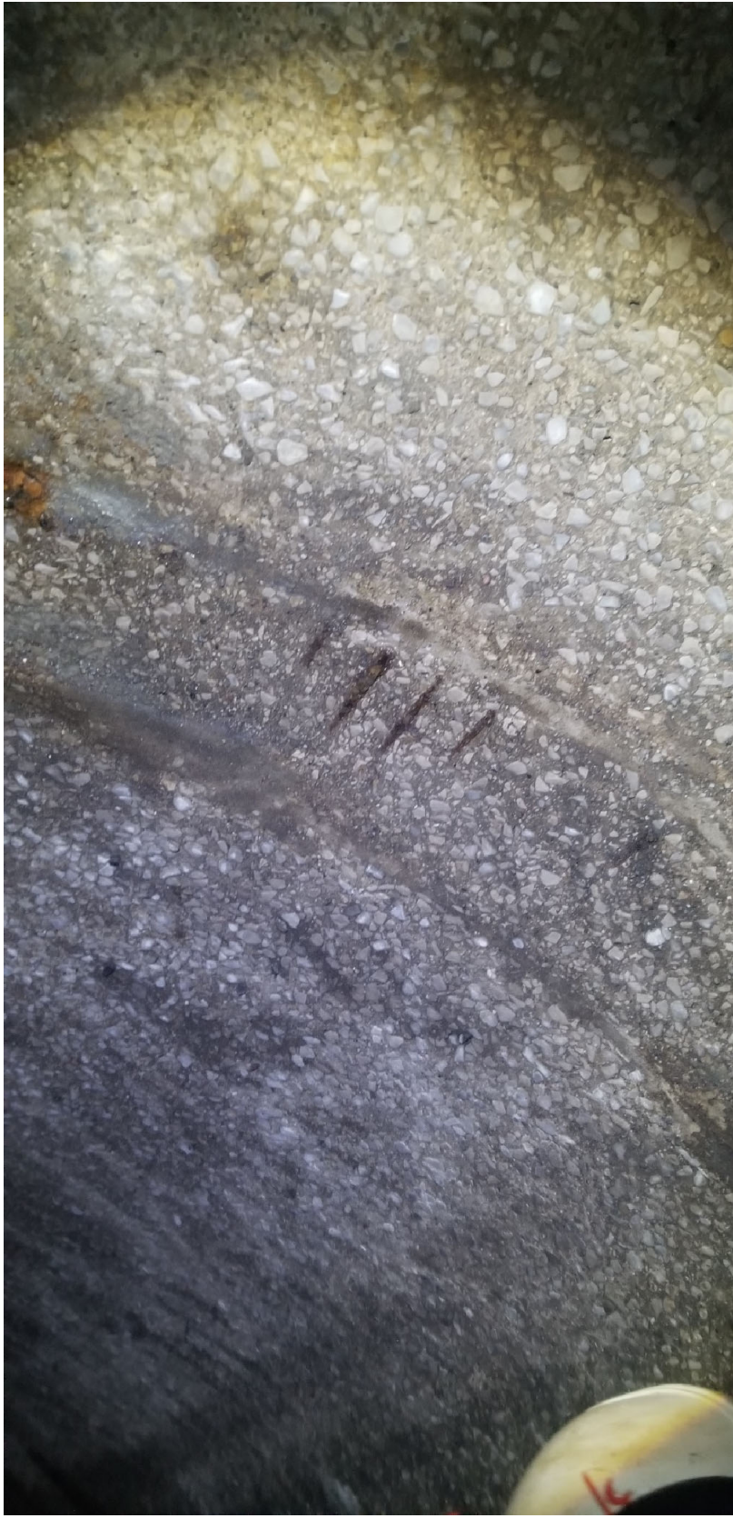
Figure 2 - Exposed Rebar in PCI-37
