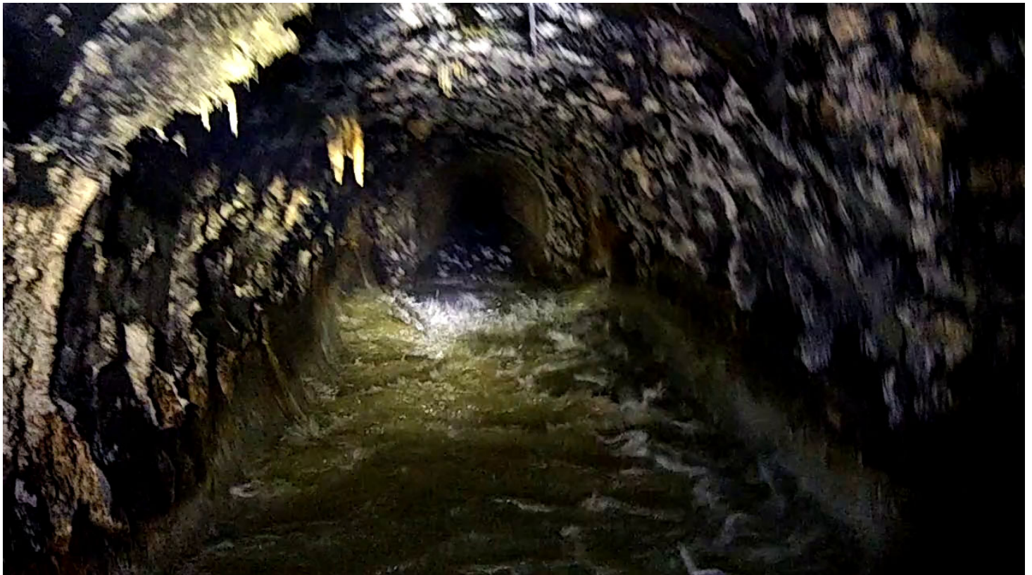
Figure 10 - Severe Deterioration in Garfield Interceptor at MA-S-2 Blind Tap
