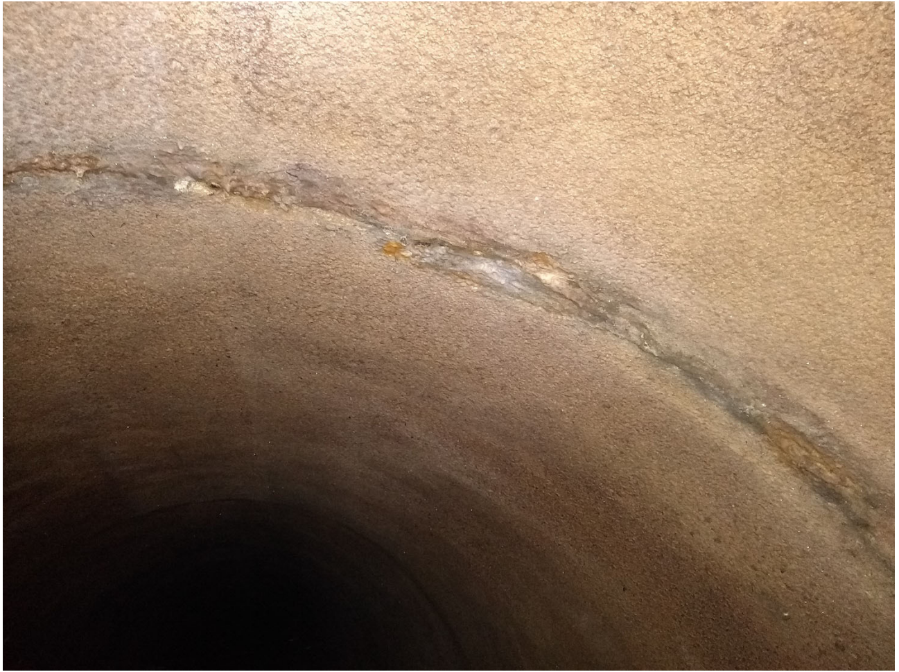
Figure 9 - Typical Infiltration in this Area
