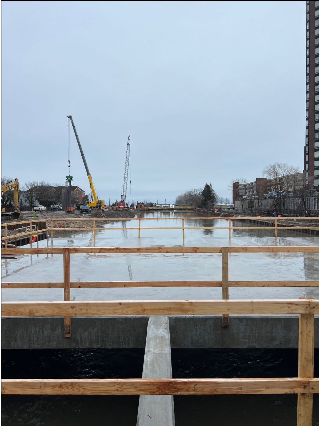
Figure 17 – Z Contractors performing upland work despite canal being flooded
