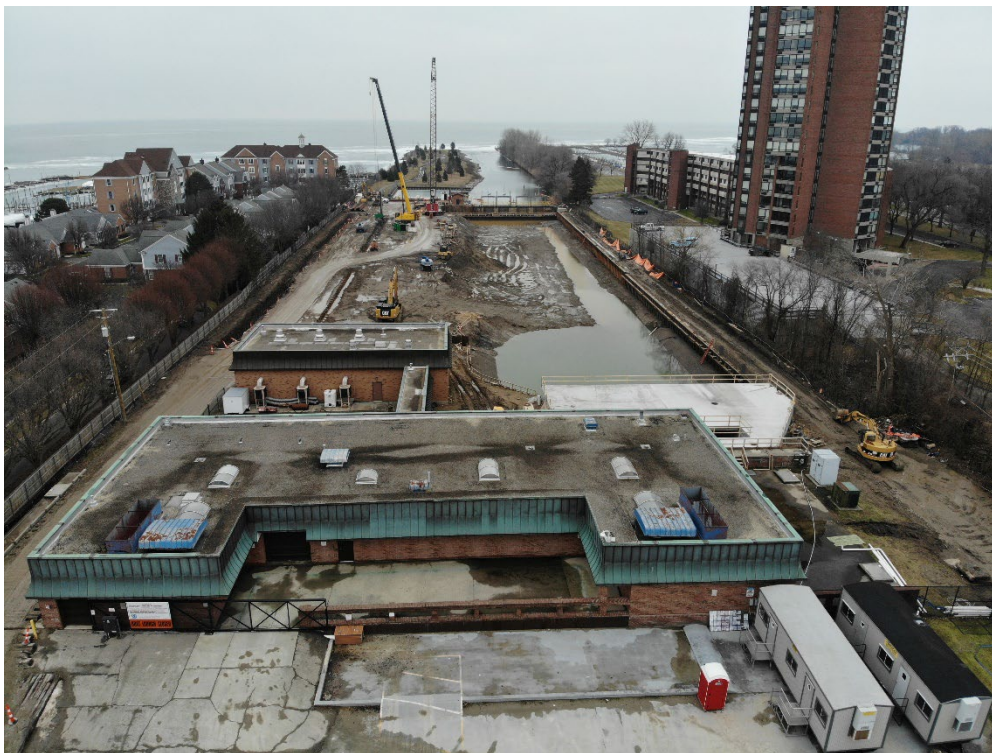
Figure 19 – Drone Aerial at 100 FT Facing East (02/01/24)-Note future canal footprint on left
