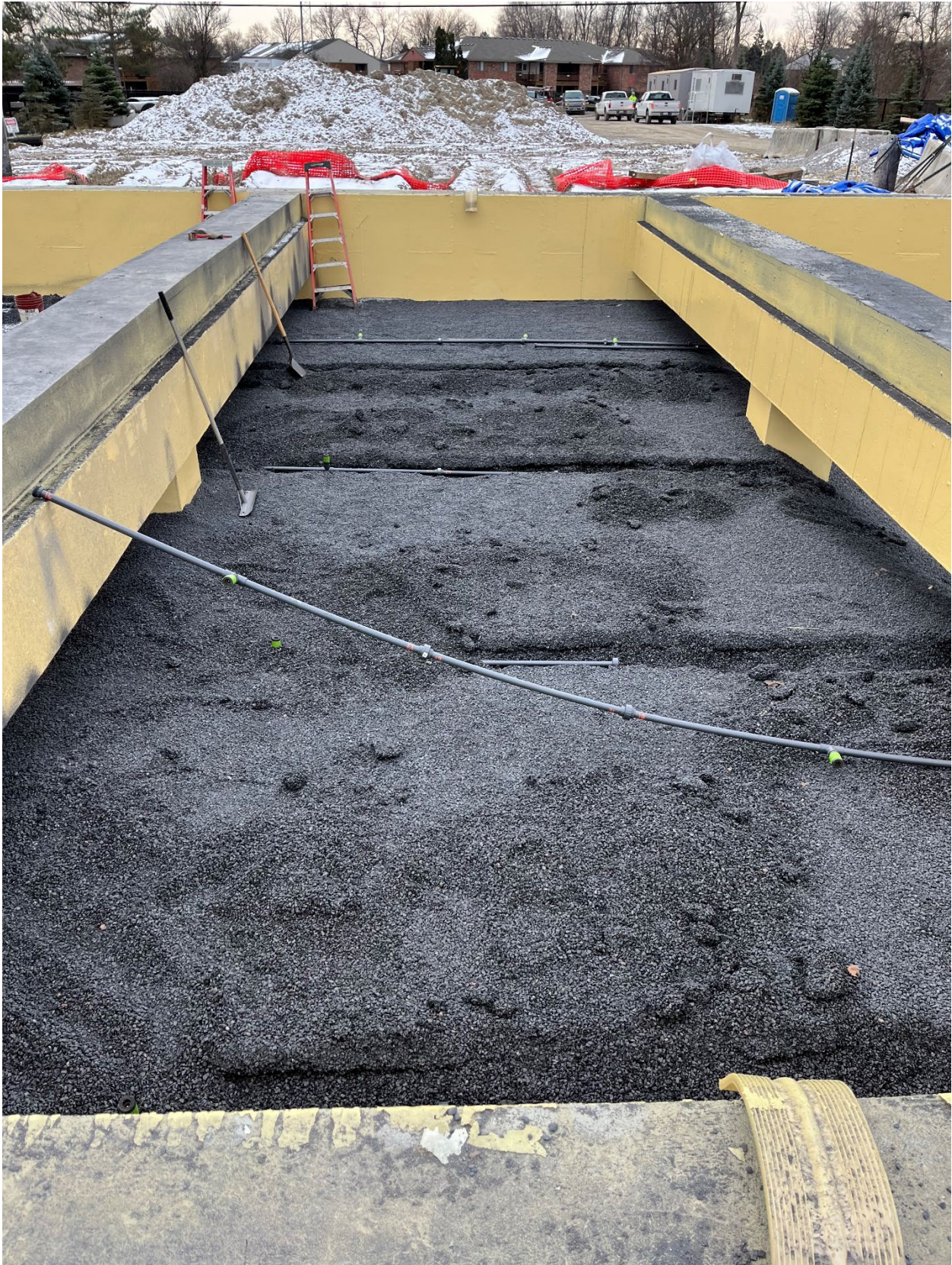
Figure 21 – Fraser Bio-Filter with Carbon Media & Water Piping
