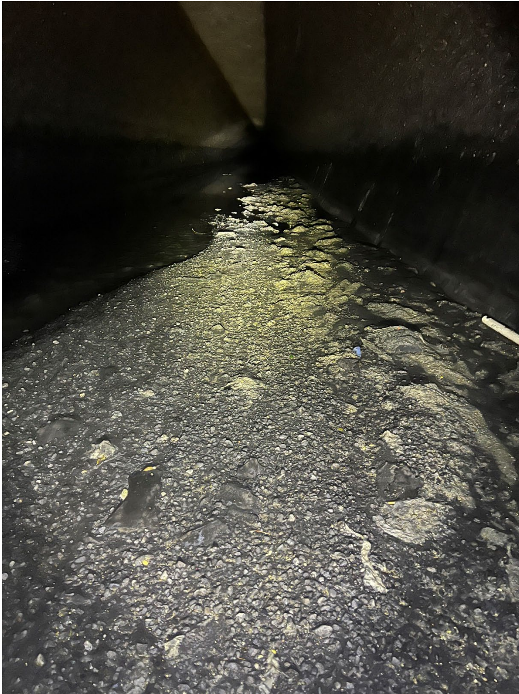
Figure 10 – RAI Curve Sediment & Debris
