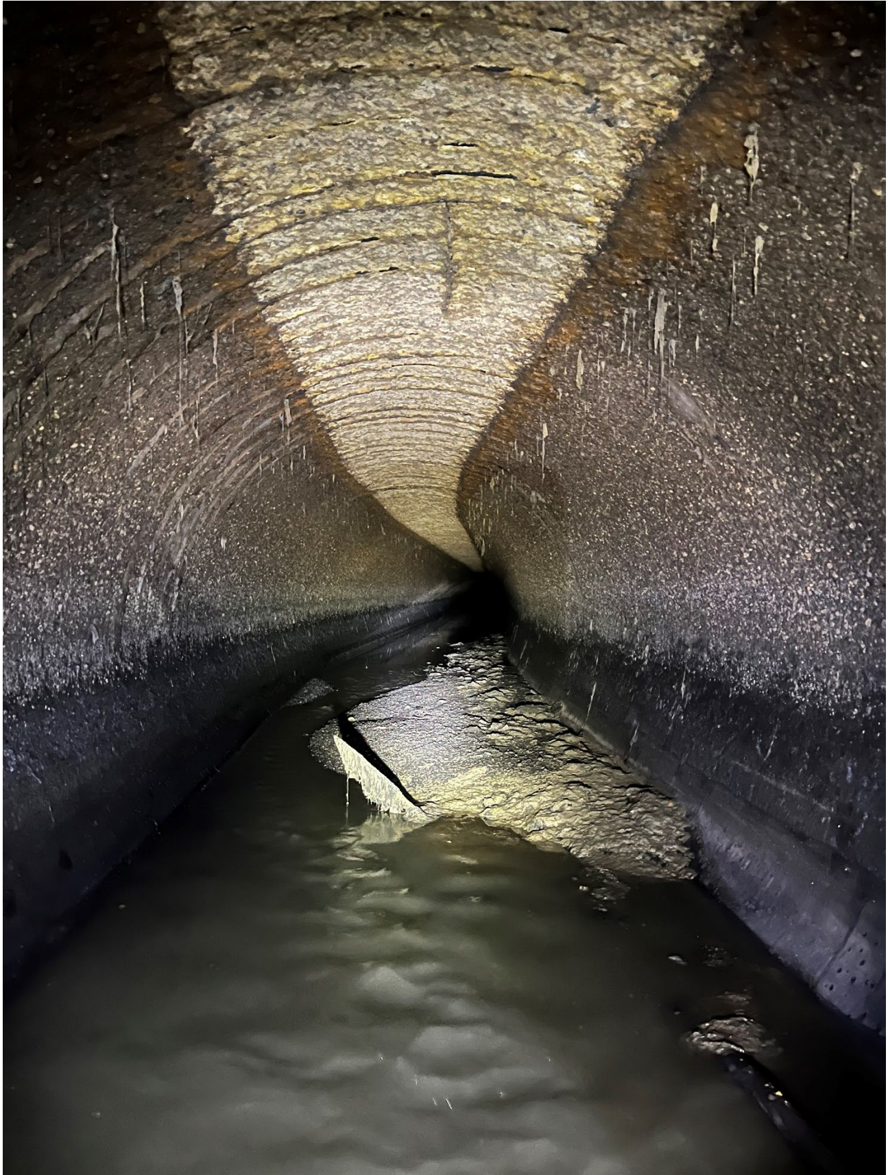
Figure 12 – RAI Curve Sediment, Debris & Condition
