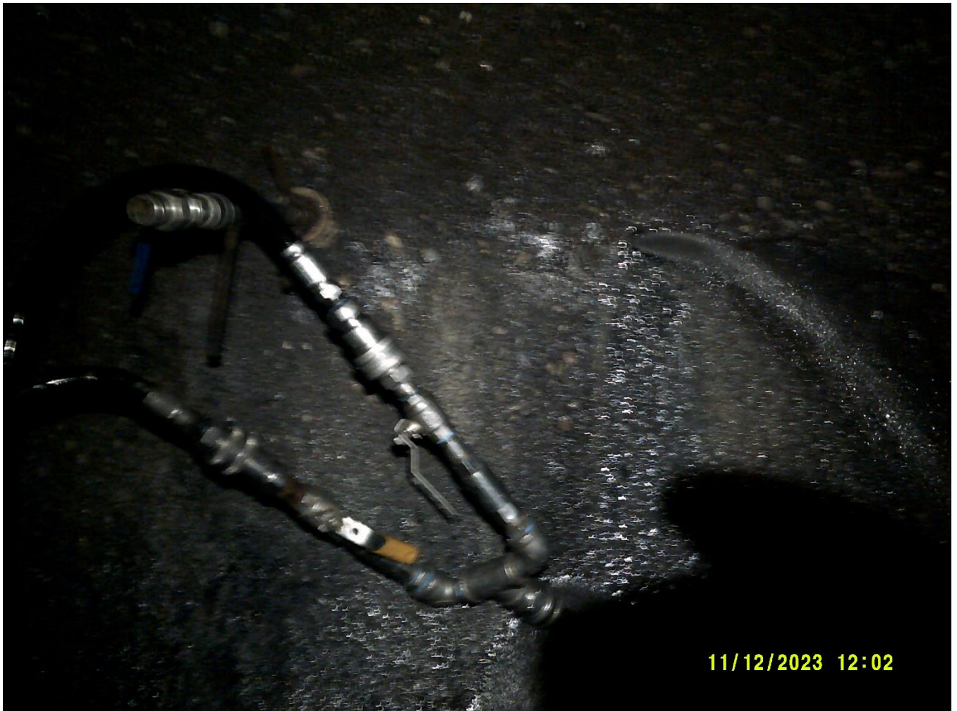
Figure 18 –Gushing Infiltration in Lakeshore Interceptor
