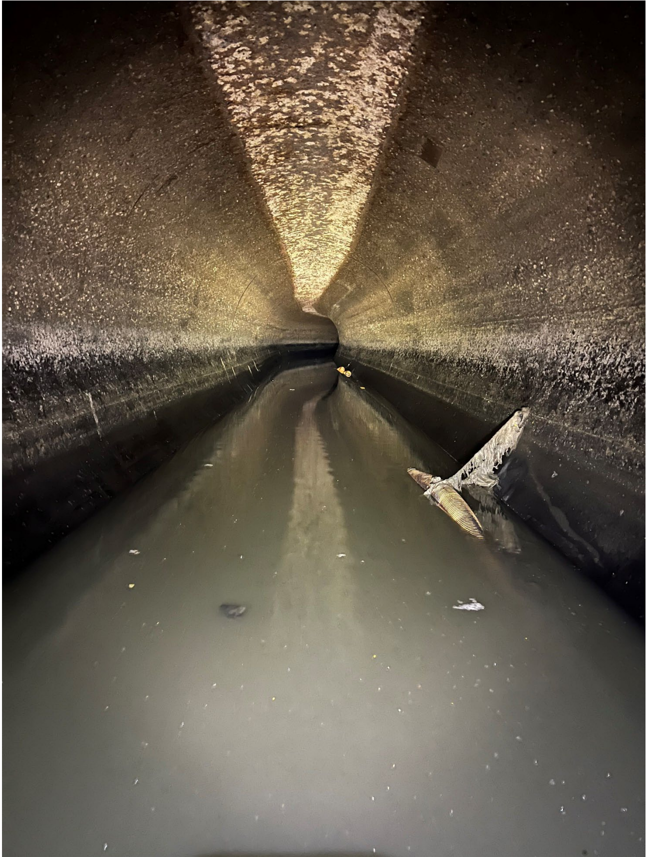
Figure 14 – RAI Curve Sediment, Debris & Condition
