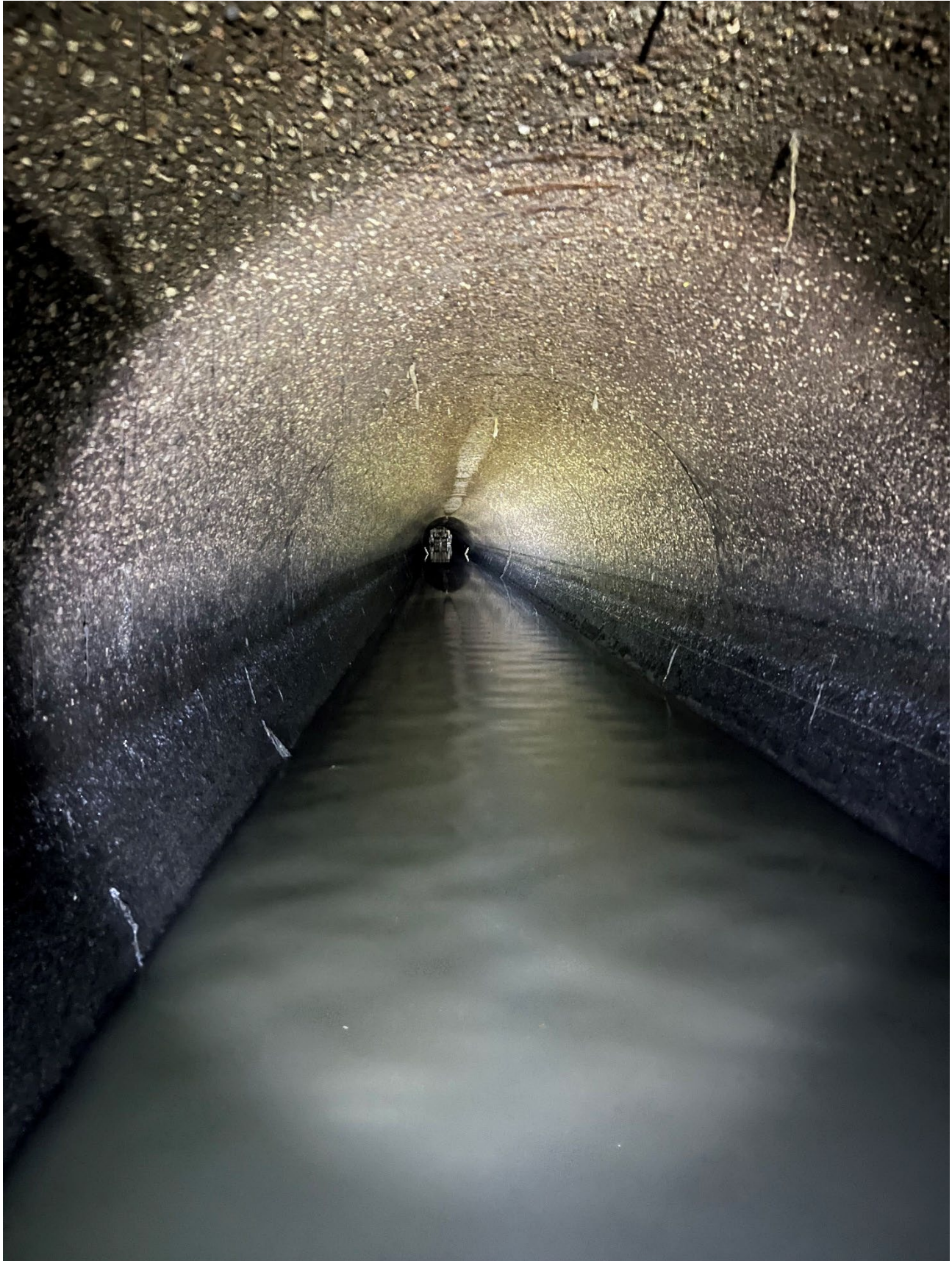
Figure 15 – RAI Curve Sediment, Debris & Condition
