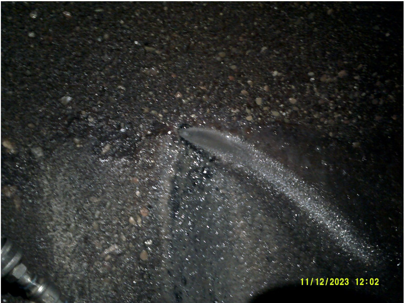
Figure 17 –Gushing Infiltration in Lakeshore Interceptor
