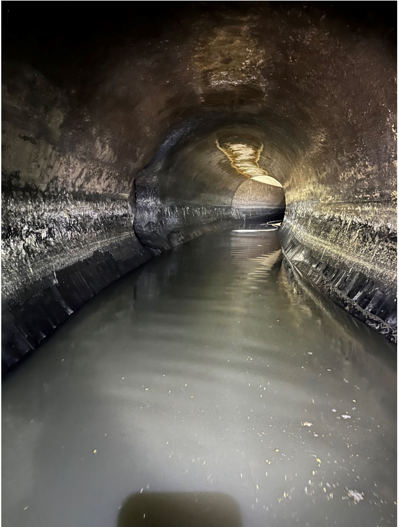
Figure 13 – RAI Curve Sediment, Debris & Condition
