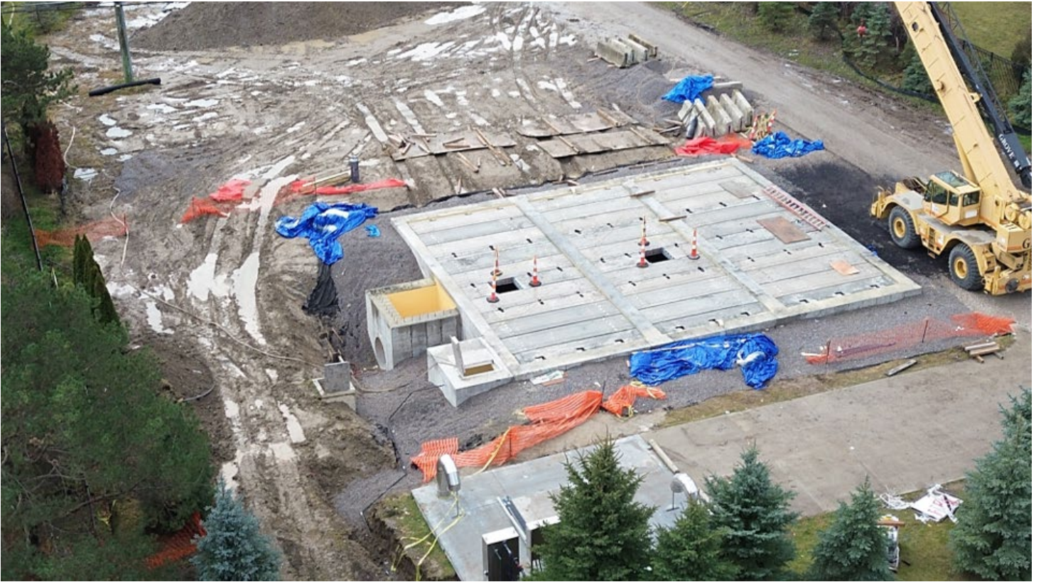
Figure 19 – Aerial View of the Fraser Biofilter
