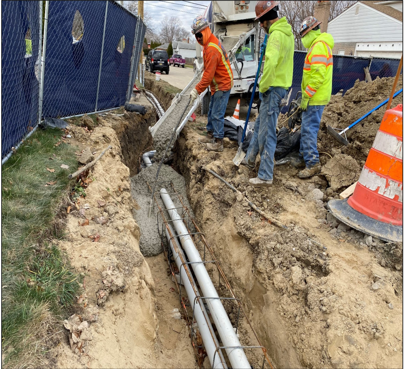
Figure 5 – Beaconsfield Control Building Concrete Duct Bank
