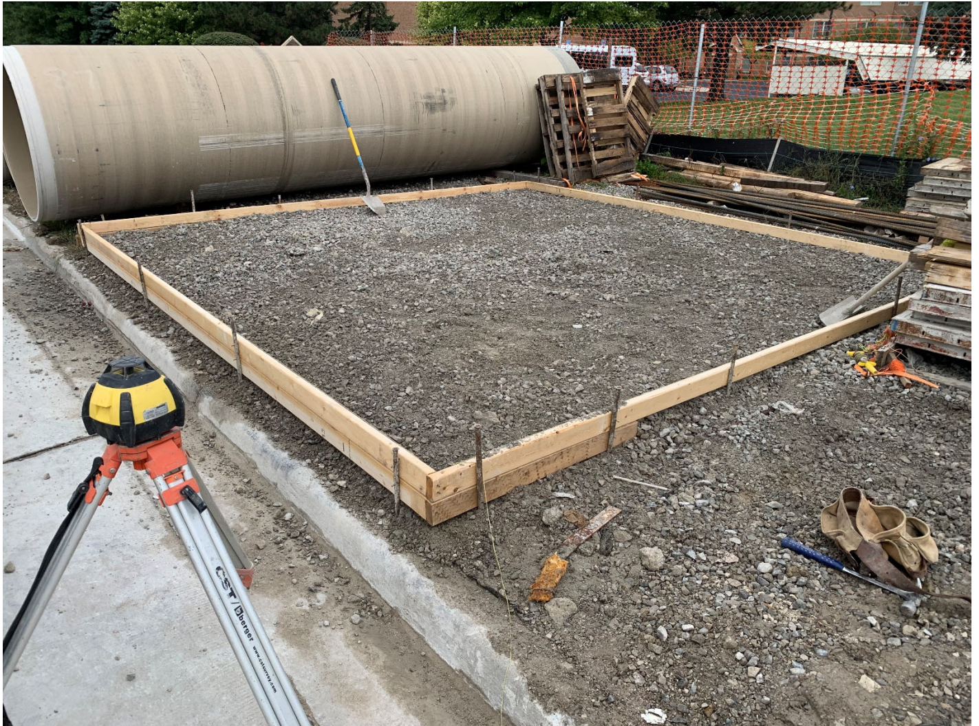
Figure 11 - CS-13 Equipment Pad
