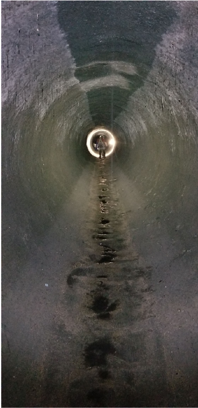
Figure 6 - PCI-37 Completely Dewatered
