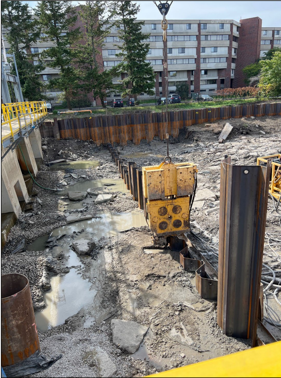
Figure 13 – New Outfall Structure Sheet Piling in foreground; new south-side sheeting in background
