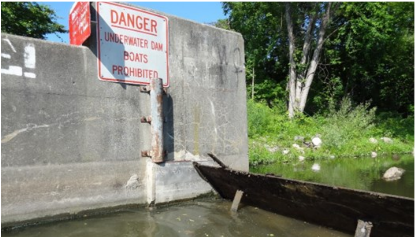
10. Minor map cracking and efflorescence observed on exterior corner of west abutment wing wall (looking west)
