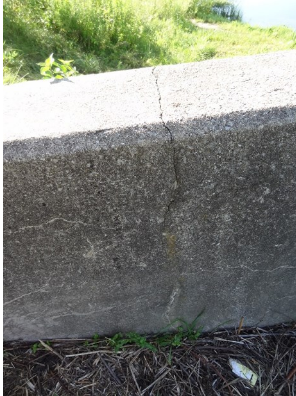
5. Vertical shrinkage cracking observed on exterior face of east abutment retaining wall (looking south)
