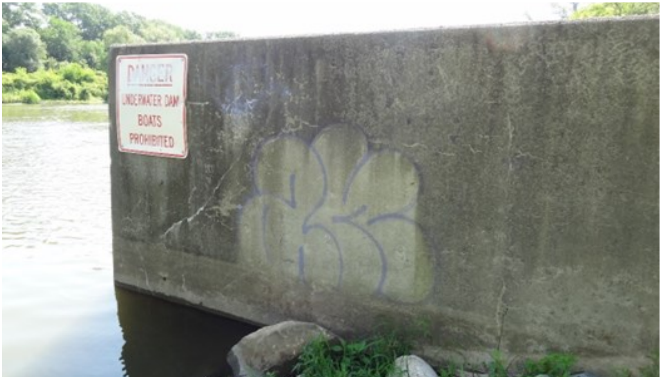
14. Minor map cracking and efflorescence observed on exterior face of west abutment retaining wall (looking south)
