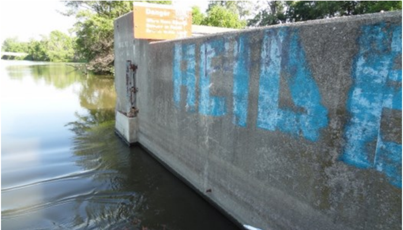
7. Vertical shrinkage crack observed on exterior face of east abutment wing wall (same crack as Photo 5; looking north)
