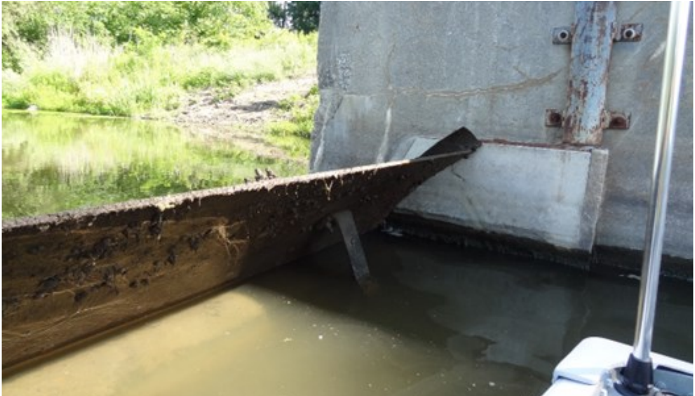
17. Termination of the weir diaphragm plate at the east wing wall showing a minor leak (looking east)
