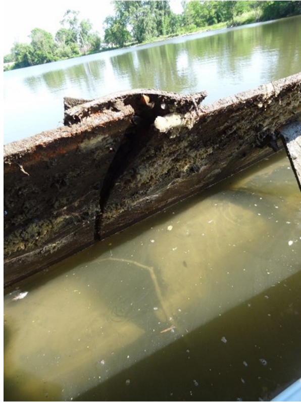
19. Uneven opening and plate bowing observed at some locations
