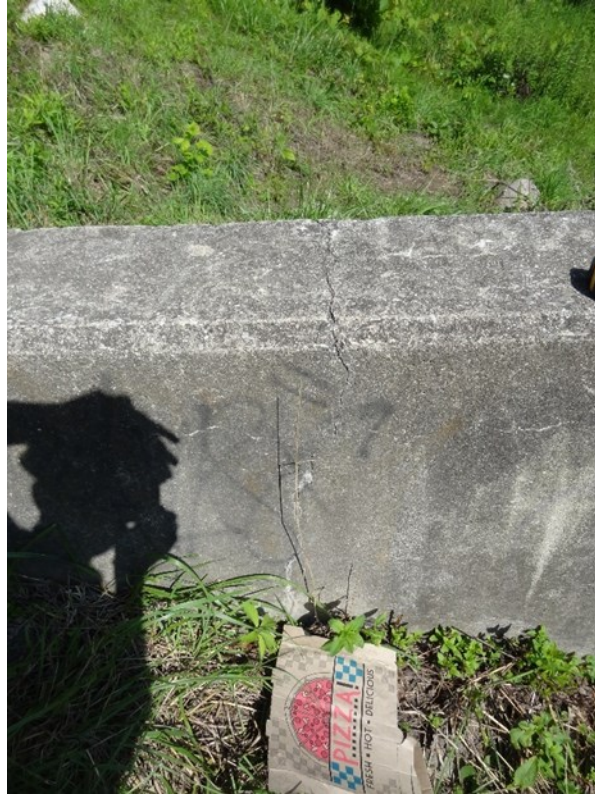
11. Vertical shrinkage crack observed on west retaining wall (looking north)
