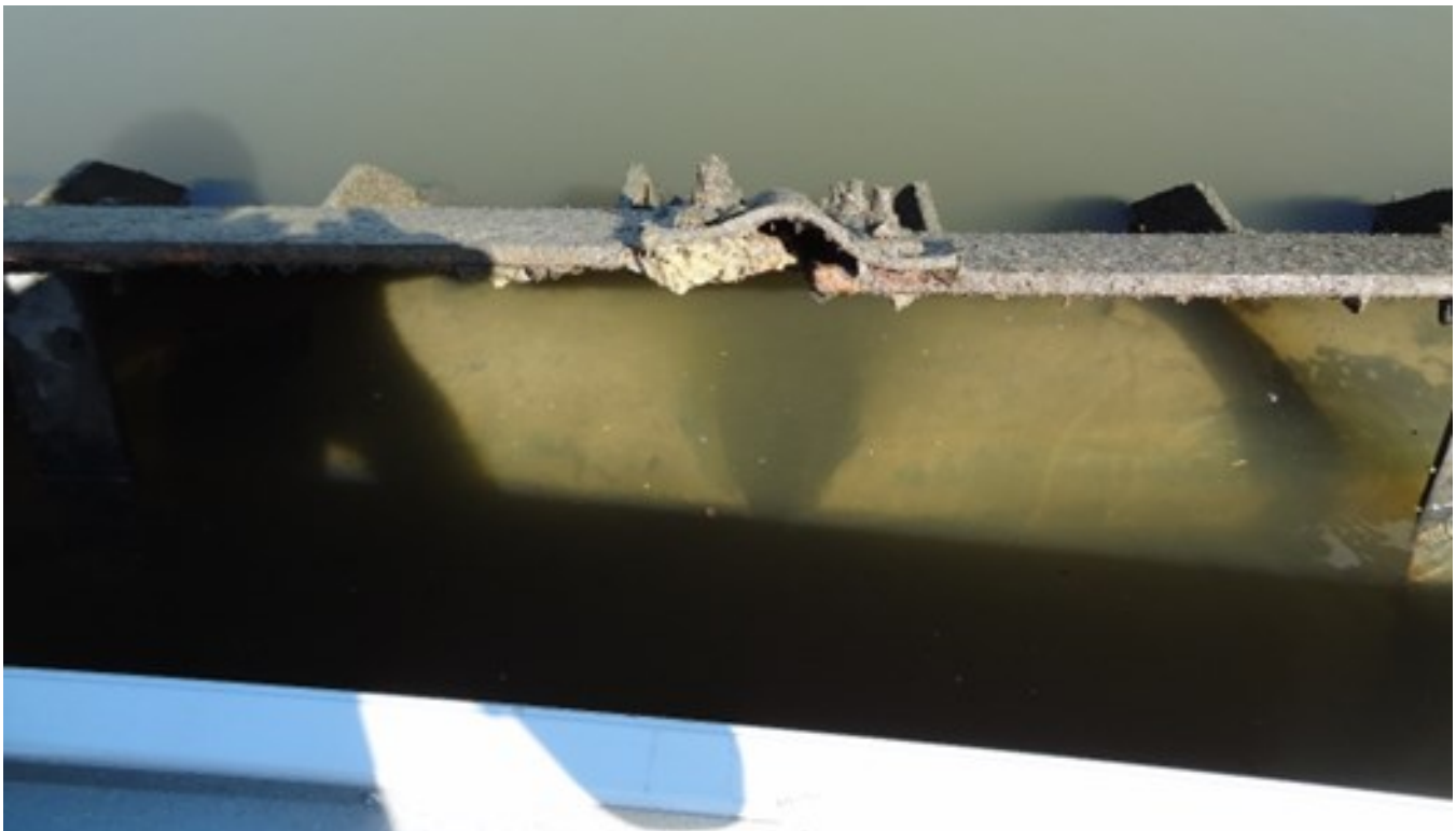
18. Rubber gasket between two plates (looking down)
