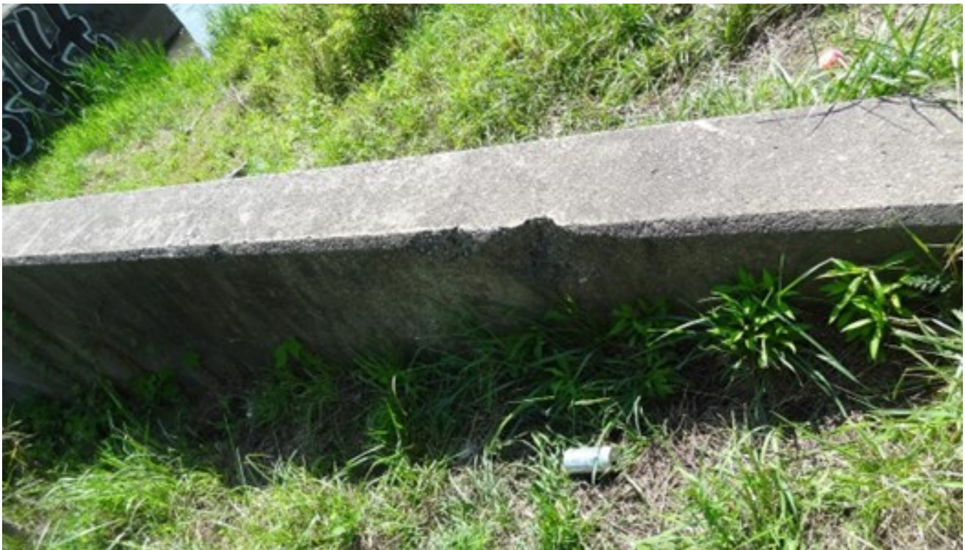
12. Minor spalls observed on the exterior face of the west retaining wall (looking south)
