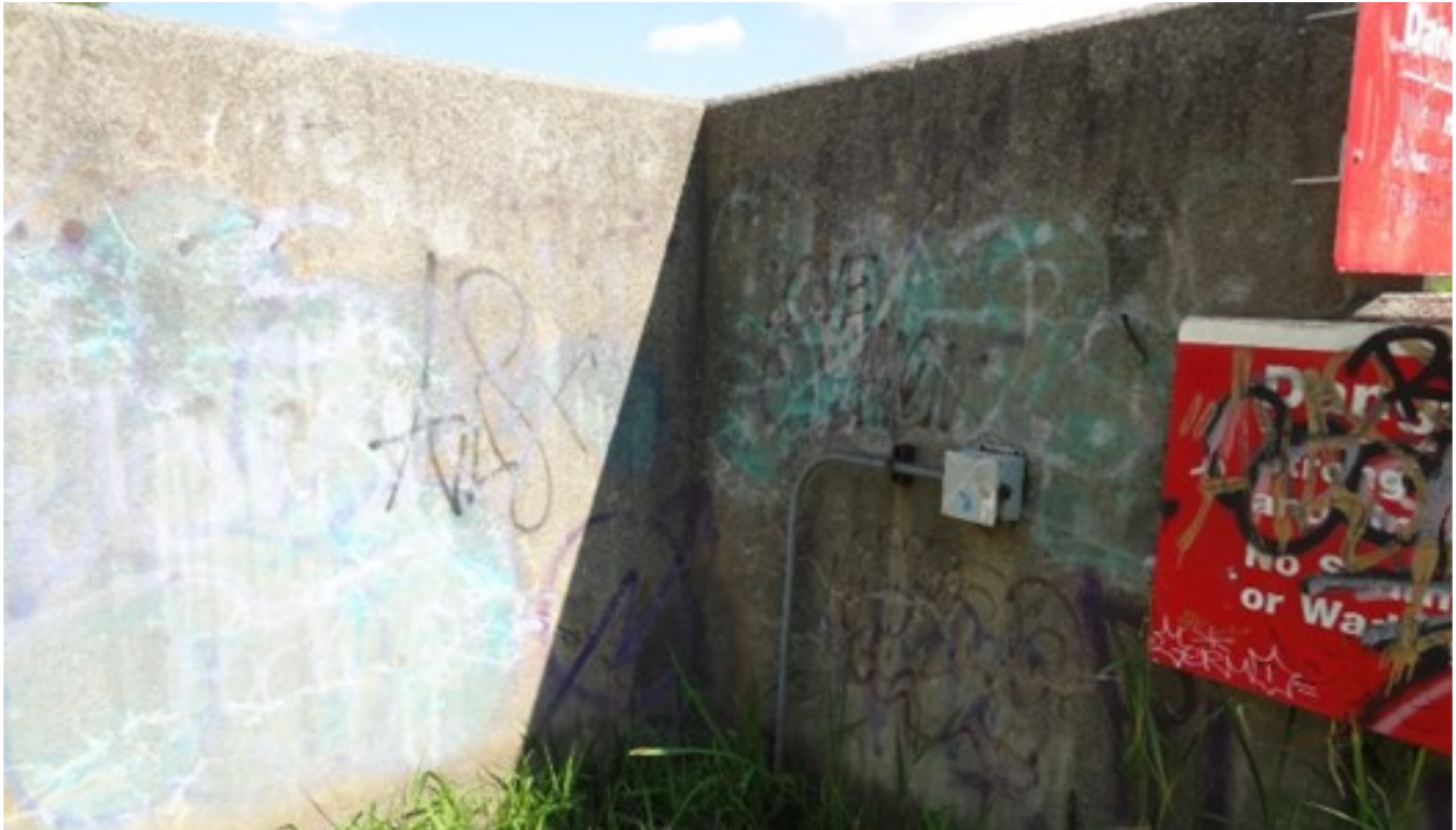
15. Minor map cracking and efflorescence observed on interior face of west abutment corner (looking north)
