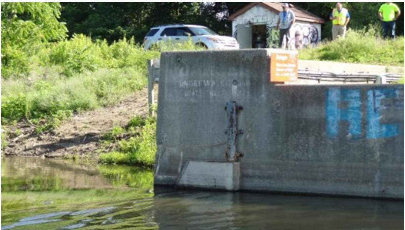
8. Map cracking and efflorescence with a shallow corner spall observed on the exterior face of east abutment wing wall (looking east)
