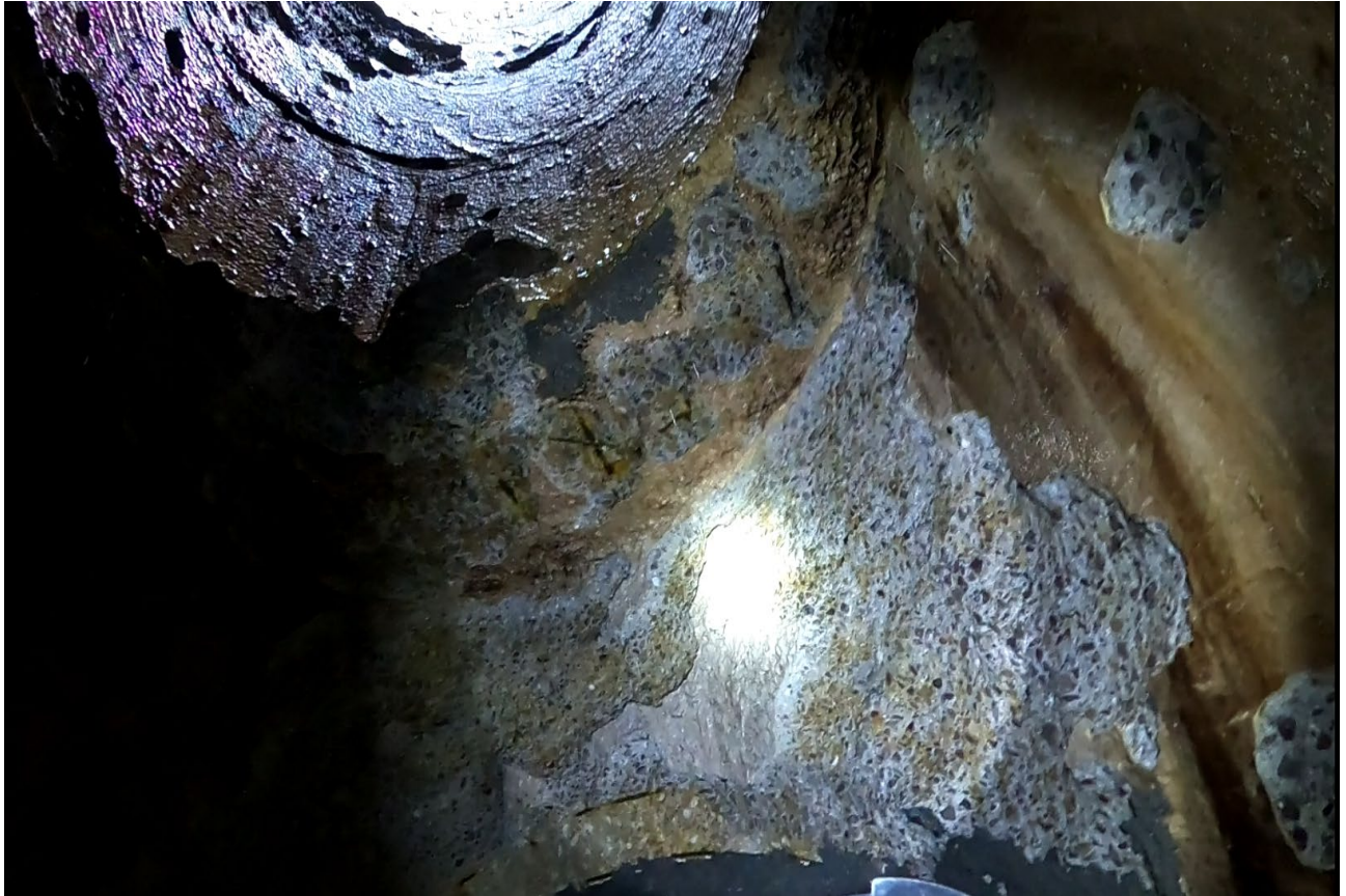
Figure 13 – SY-S-3 (West Side) Severe H2S Damage
