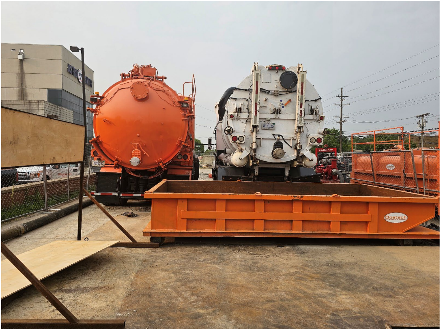
Figure 7 – Sediment/Debris Removal Equipment at CS-2
