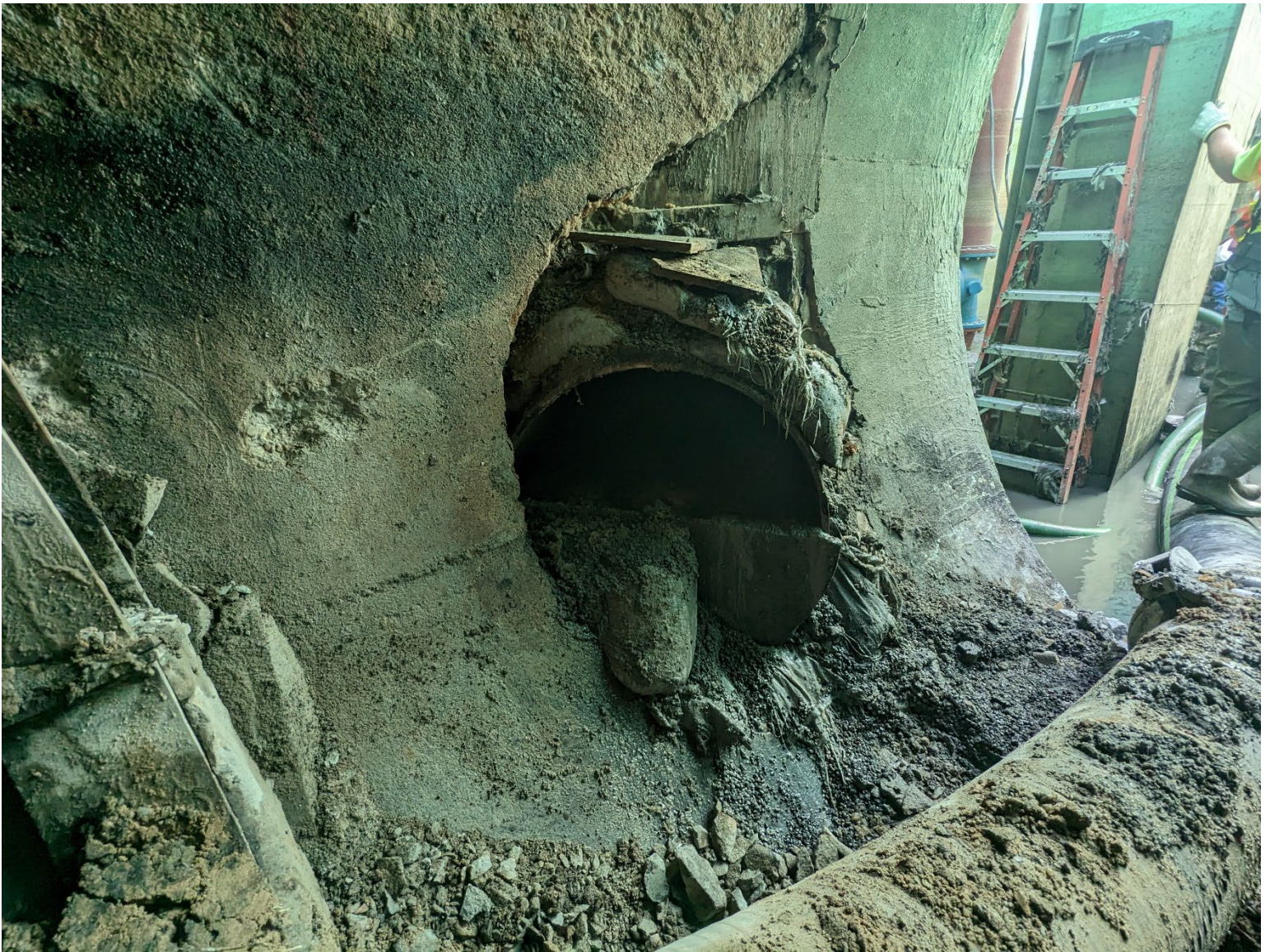
Figure 3 – Drop-Pipe Casing at Southwest Discharge
