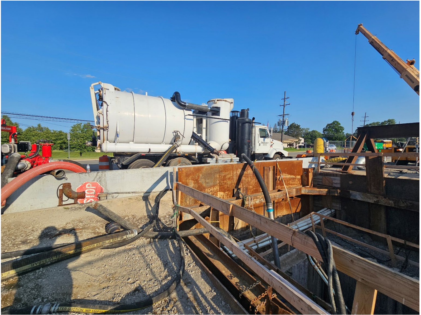
Figure 8 – Sediment/Debris Removal Equipment at CS-2
