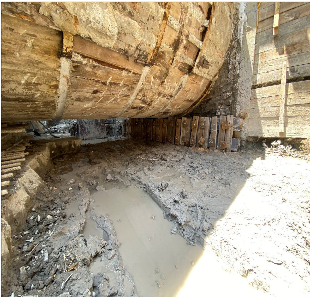
Figure 5 – Tunnel Undermining @ West Wall of Beaconsfield Shaft
