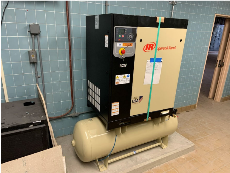
Figure 1 – New air compressor in East Building mechanical room
