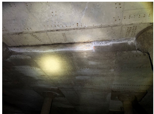
Figure 7 – Ceiling crack / damage area after demolition
