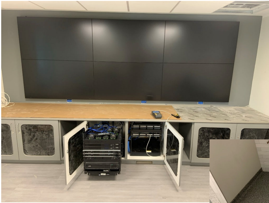
Figure 2 – SCADA Video Wall (Abel Electronics)
