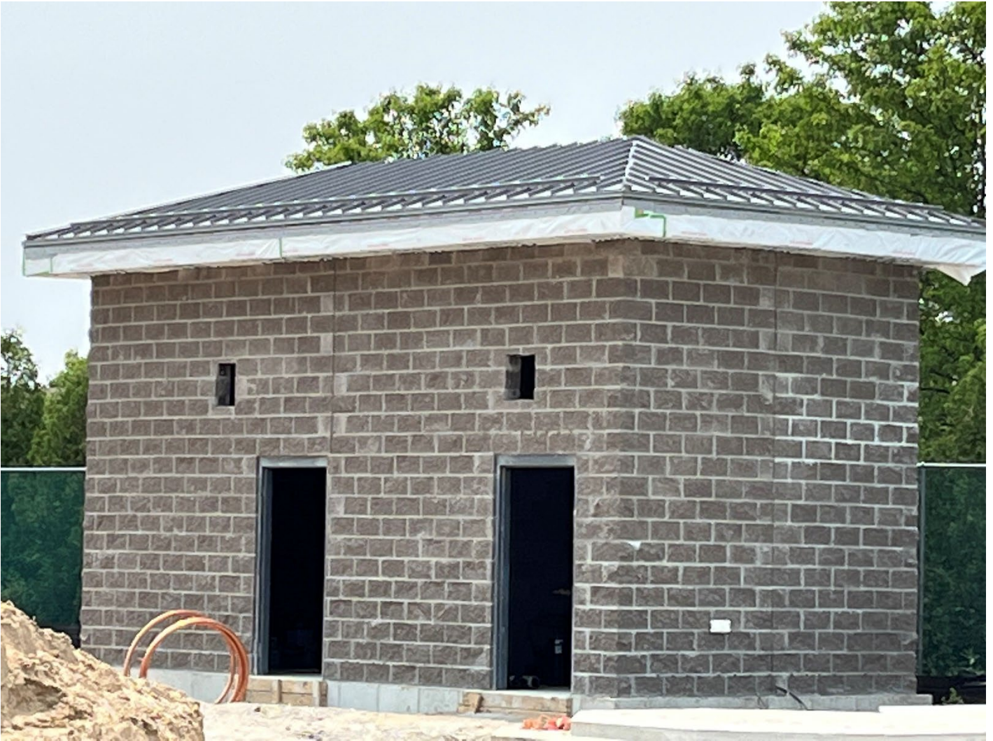
Figure 12 – NGI PS Odor & Corrosion Equipment Building
