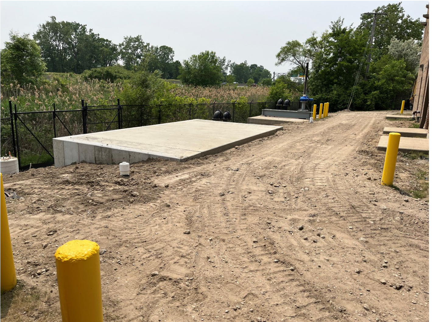
Figure 13 – CPS Equipment Pad
