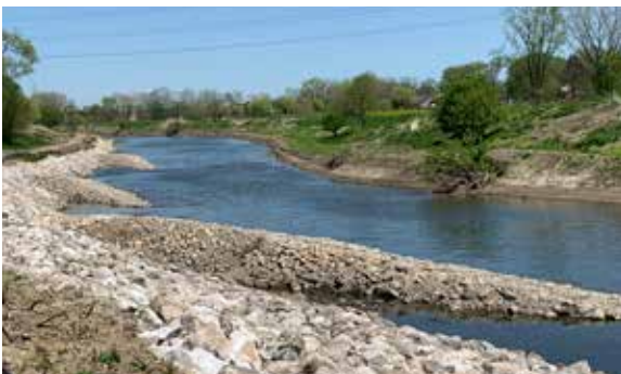
During strong or higher flow, especially after heavy rain, the three completed “J-hooks” at the Red Run Drain work in unison to prevent erosion of the drain bank by directing the flow toward the center of the channel.
