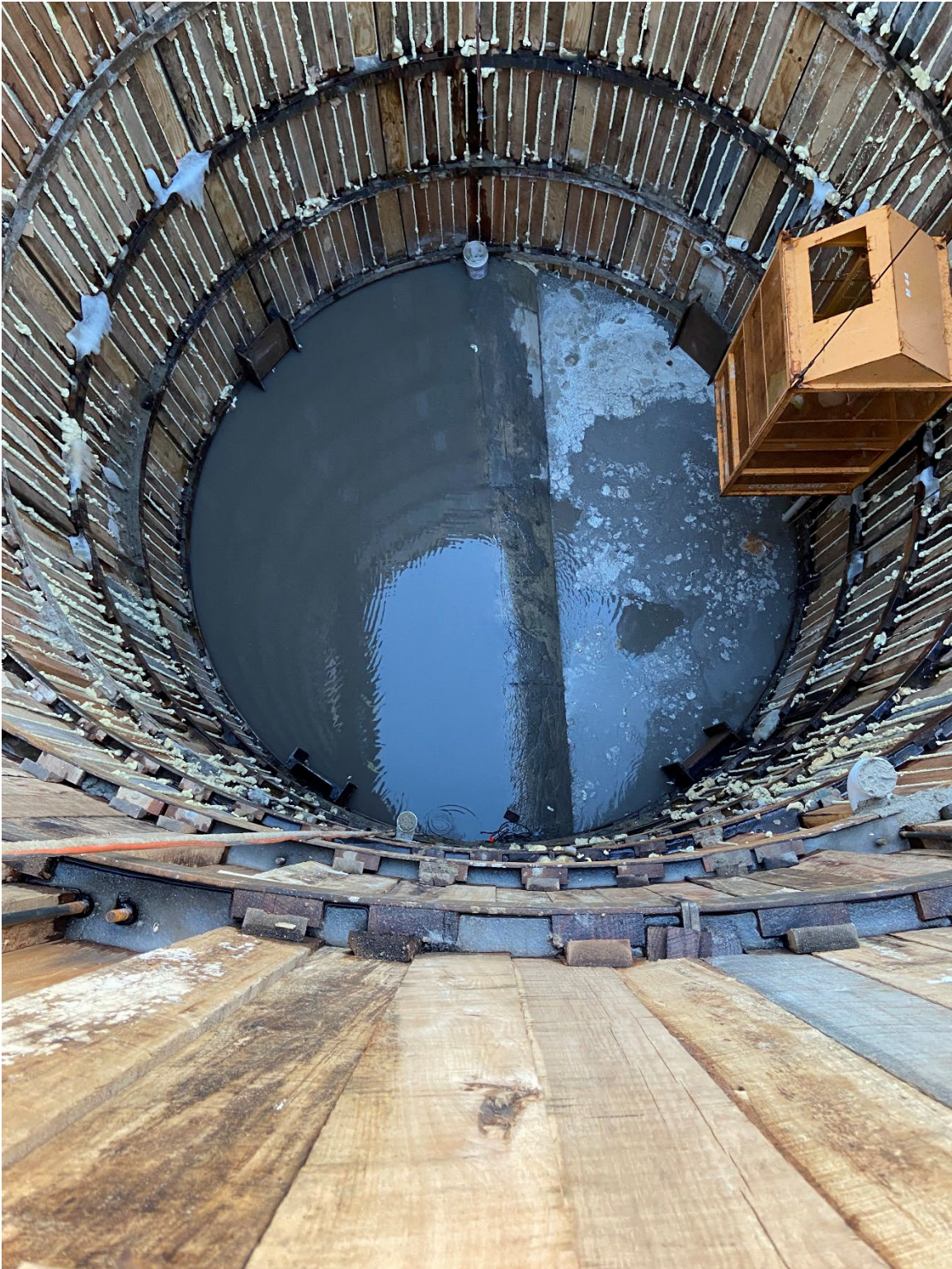
Figure 11 – Lining Completion Shaft Flooded
