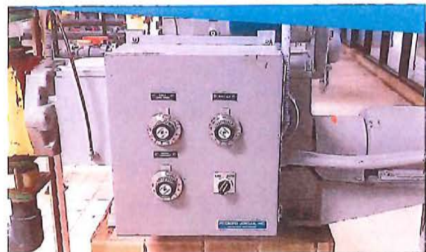
The chemical feed pumps at both Chapaton and Martin Basins require upgrading because replacement parts are no longer available from suppliers.
