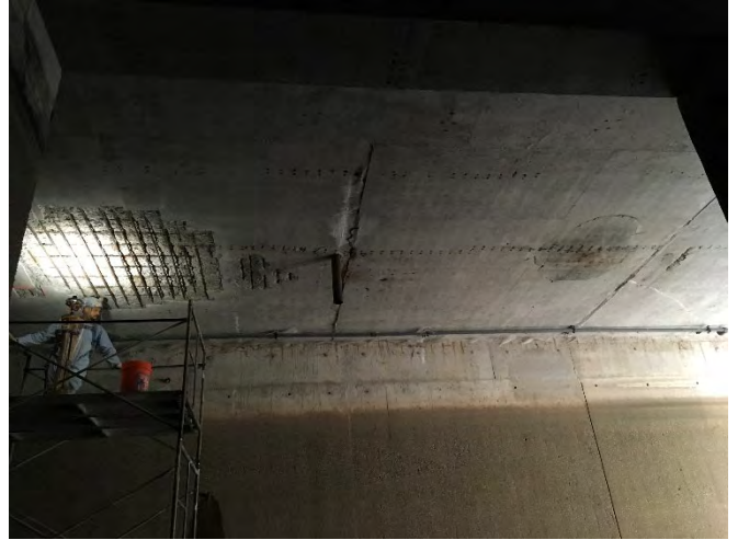
Figure 4 – Aeration Chamber – Exposed Rebar and Ceiling Repairs
