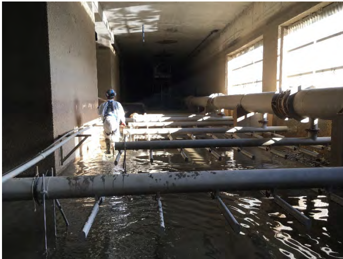
Figure 3 – Aeration Chamber – Blower Equipment & Scaffolding
