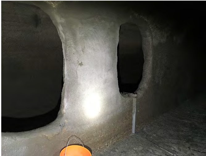
Figure 1 – 9-Mile Drain - Equalizer ports at Chapaton Station Gate
