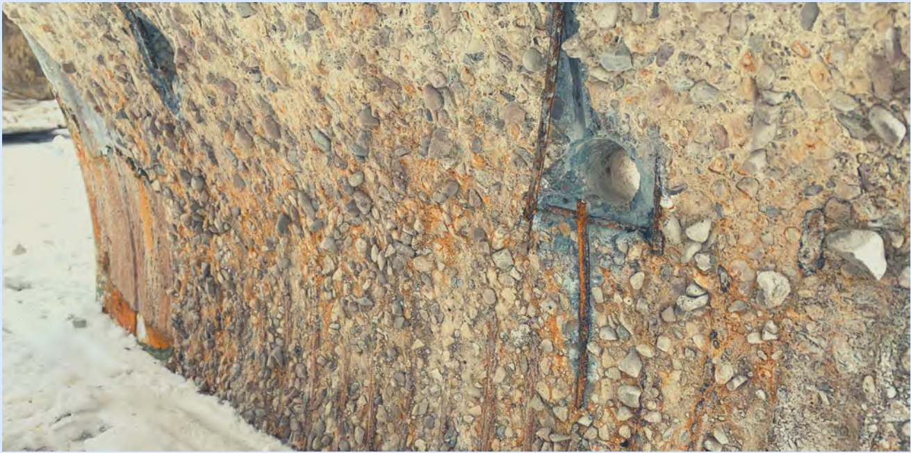
Degradation shown of removed pipe at Segment 6
