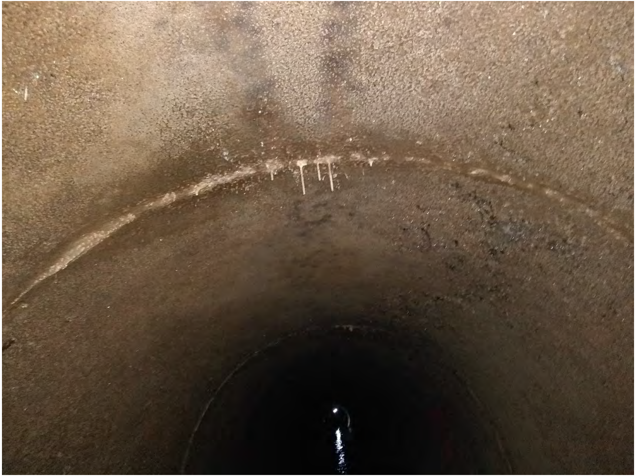
Figure 10 - Typical Infiltration in this Area
