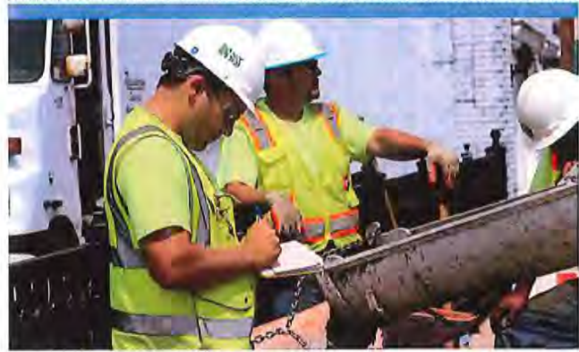
Wade Trim construction inspectors will be on site to monitor construction activities and document their progress in an Inspector Daily Report (IDR).
