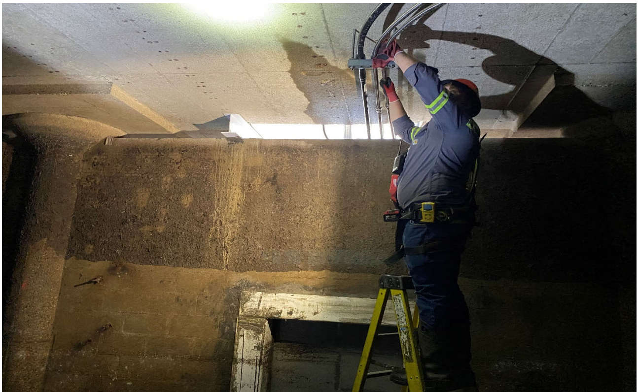
Figure 3 - New Hydraulic and Electrical Conduit for Gate Operation
