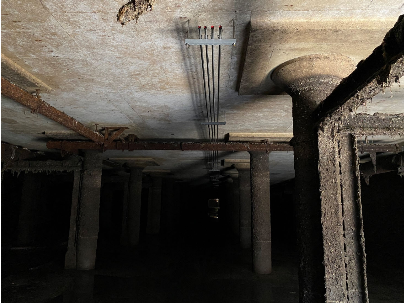
Figure 1 - Hydraulic Lines and Electrical Conduit in RTB
