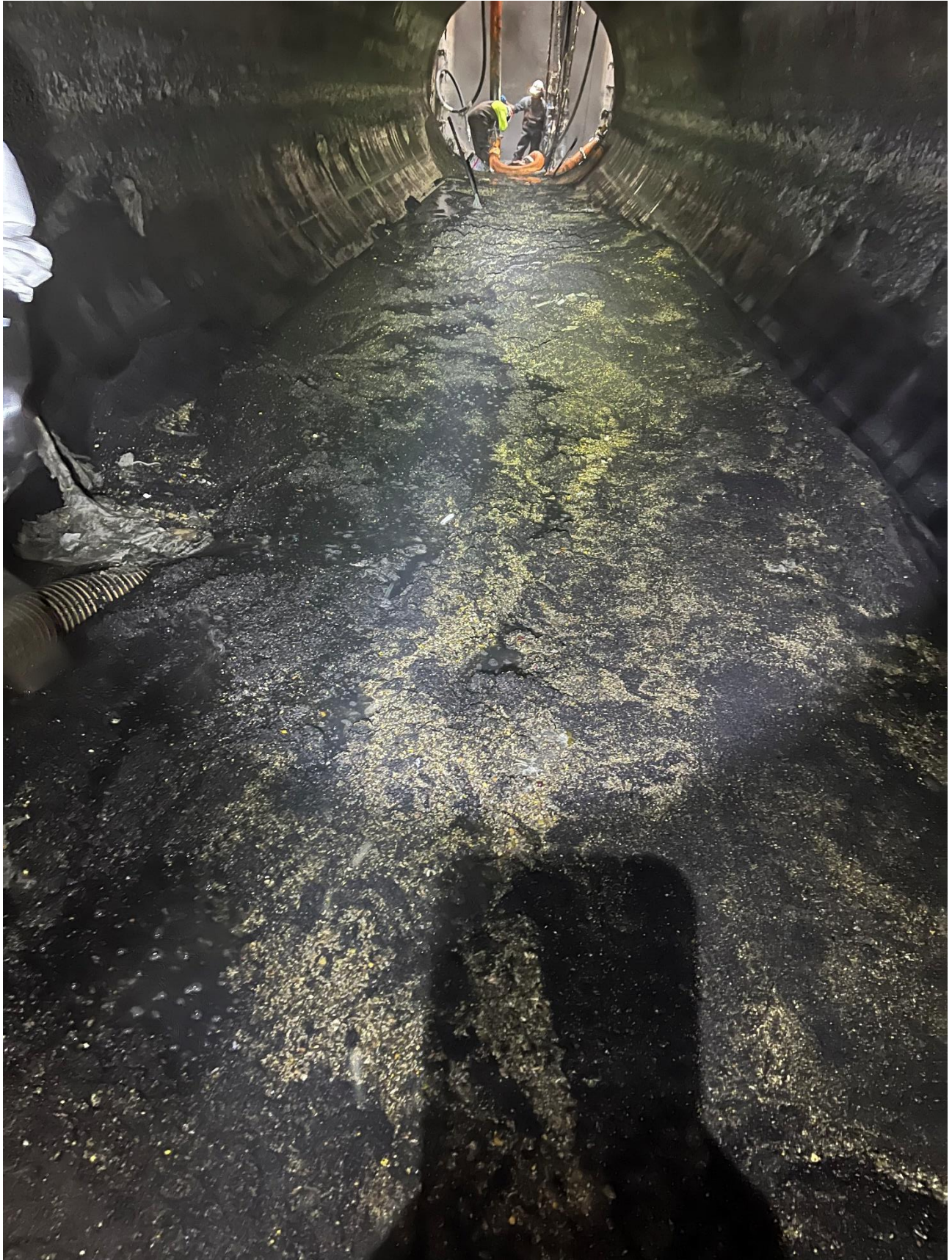
Figure 10 – Viscous Sludge at CS-2
