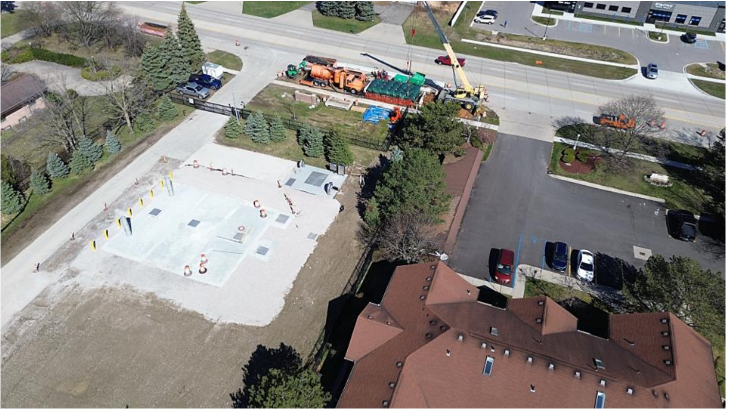
Figure 12 – Aerial View of the Fraser Biofilter
