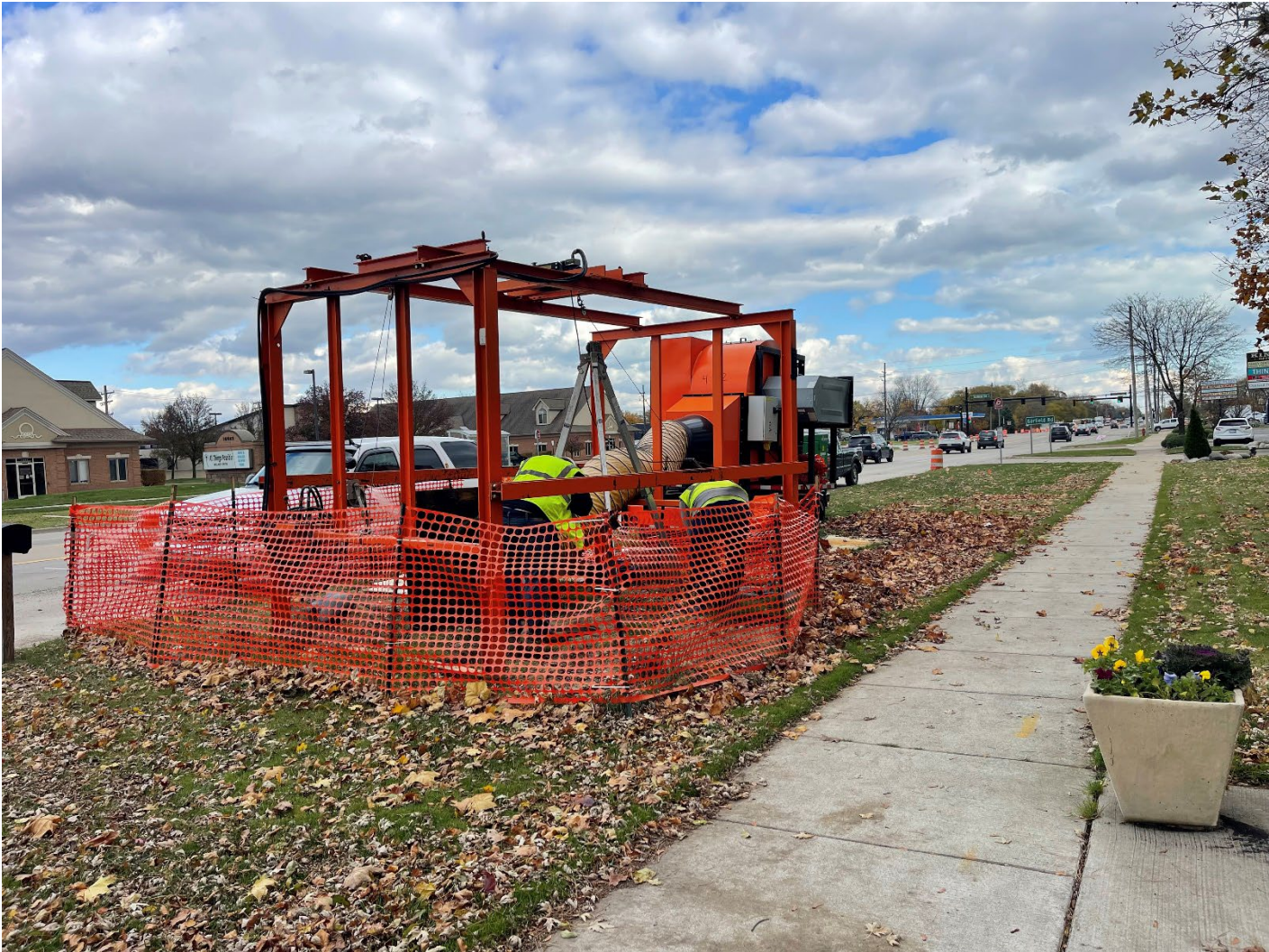
Figure 10 – MH-10 Ventilation and CSE Entry for Cleaning Operations
