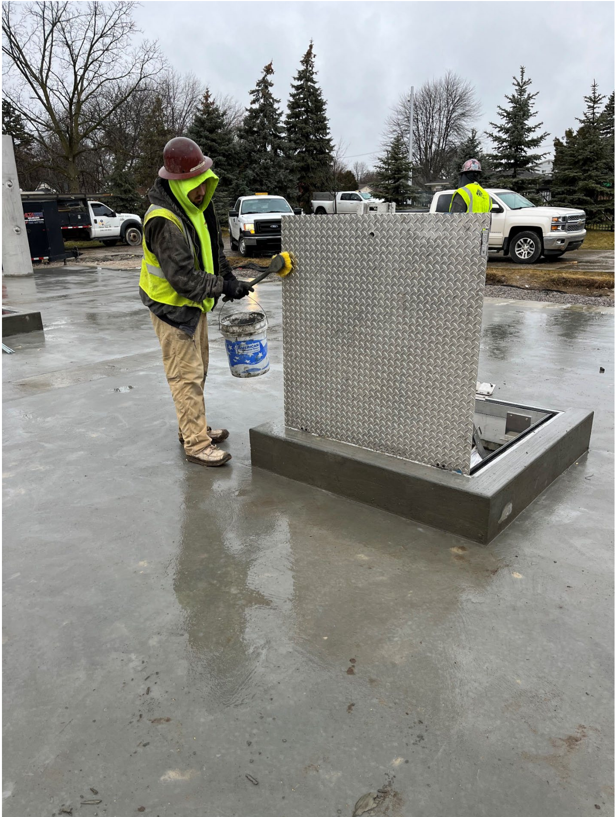
Figure 13 – Fraser Bio-Filter Access Hatch
