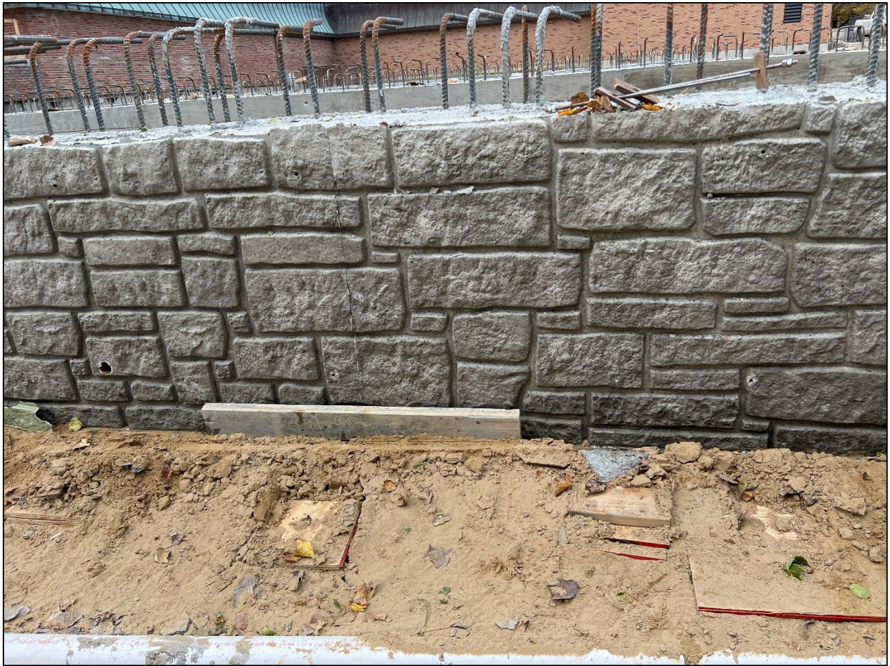
Figure 14 – Decorative stamped finish on side of screening structure (to match future sheeting cap)
