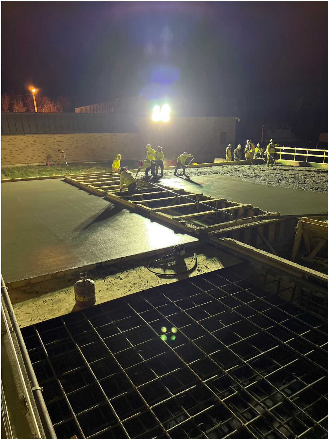
Figure 16 – Screening Structure top slab pour; north half. Poured in favorable evening weather conditions
