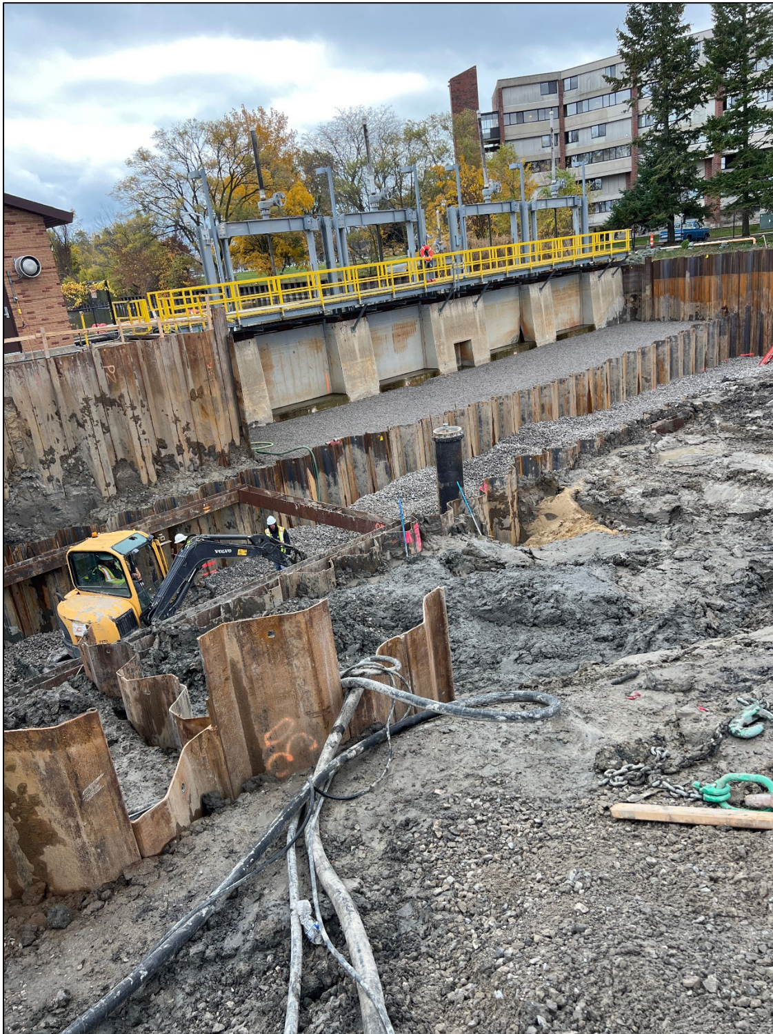
Figure 16 – Outfall Structure sheeting & stone base (right), Ex. outfall building and cofferdam (left)
