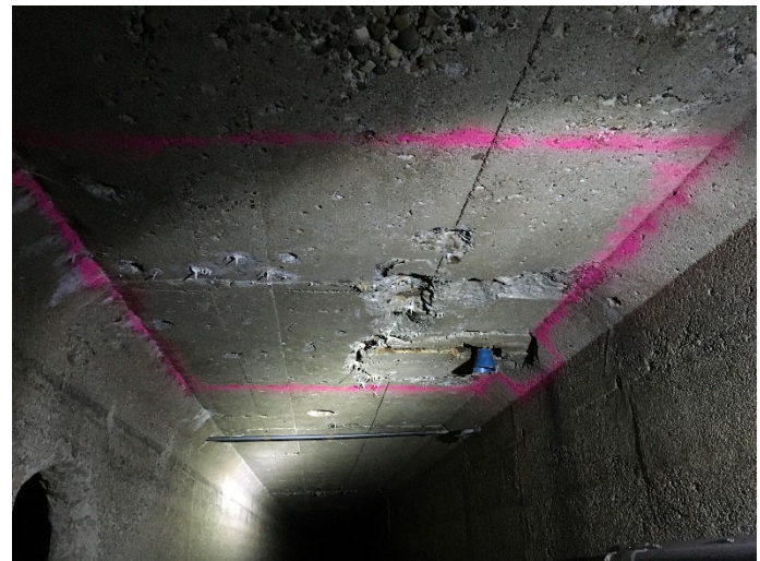
Figure 5 – Damage / delaminated area within 9-Mile Drain-North Box
