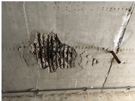
Figure 6 – Ceiling damage in Aeration Chamber-not in base scope
