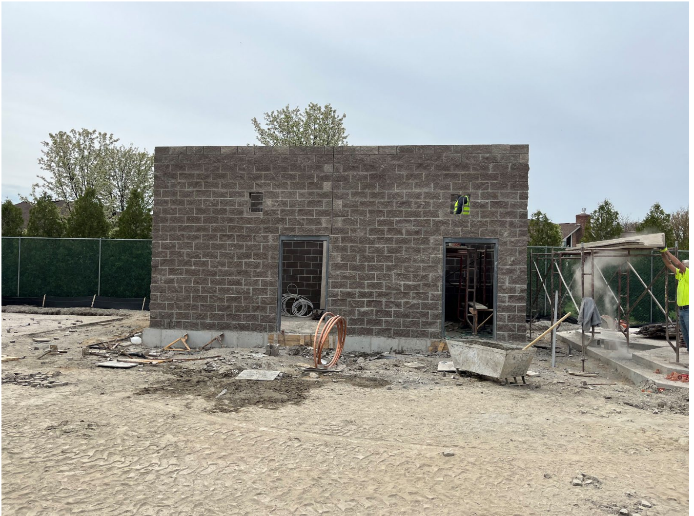
Figure 13 – NGI PS Odor & Corrosion Equipment Building
