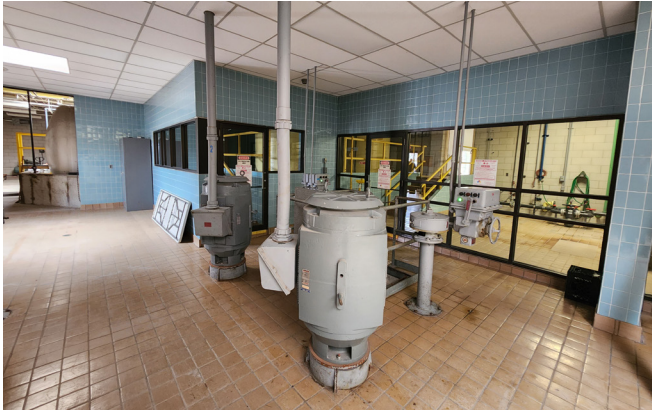
As part of our evaluation during the BOD phase, Wade Trim will look at options to remove motors and valve actuators at the floor level to provide more open space as well as better access into the pump vault below.
