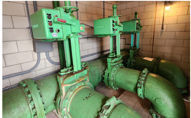
The existing knife gate valves and actuators will be replaced in kind. A new pipe spool piece from the valve to the 90-degree bend may be required due to the Victaulic connection if the new valve lay length is larger than the existing valve.
