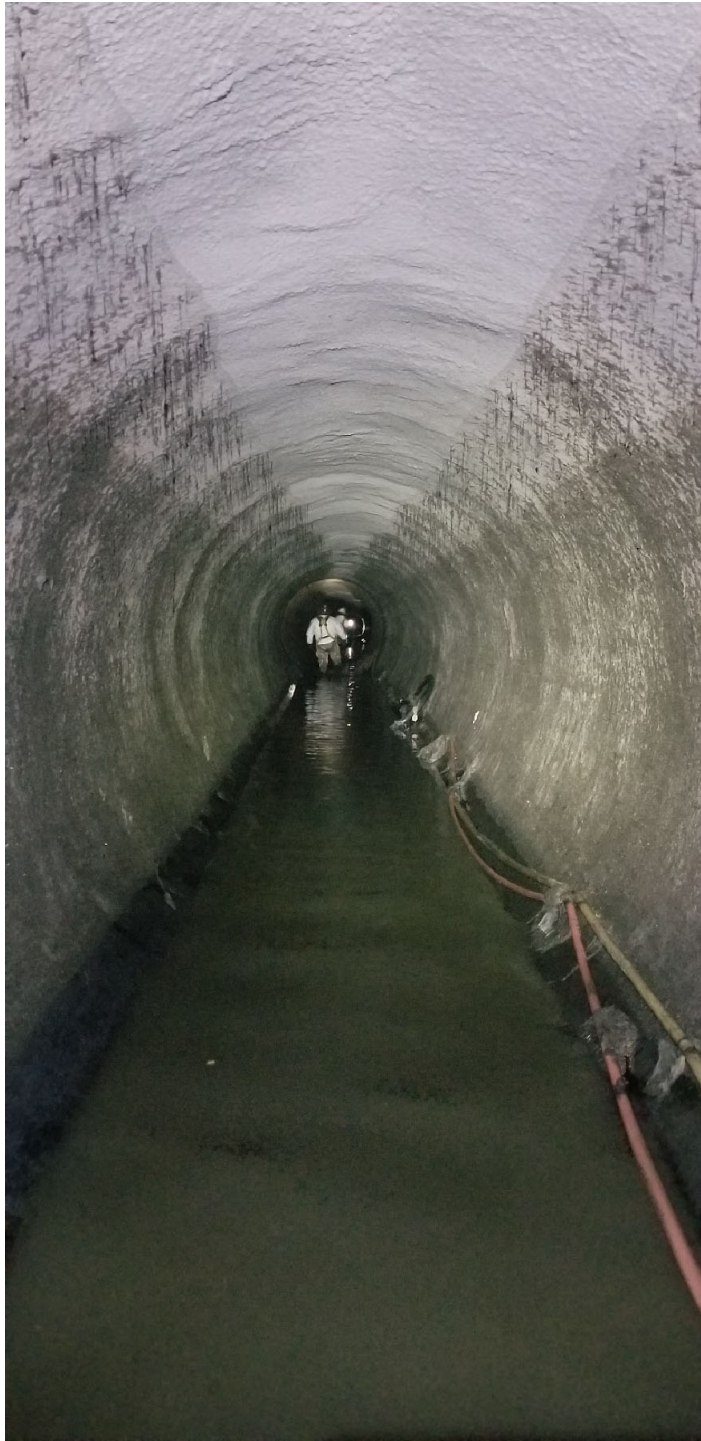
Figure 6 – Portion of the 8-foot Diameter Interceptor Spray-Lined
