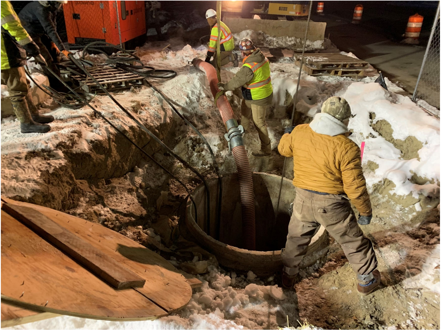
Figure 11 –RAI Flow Control Test
