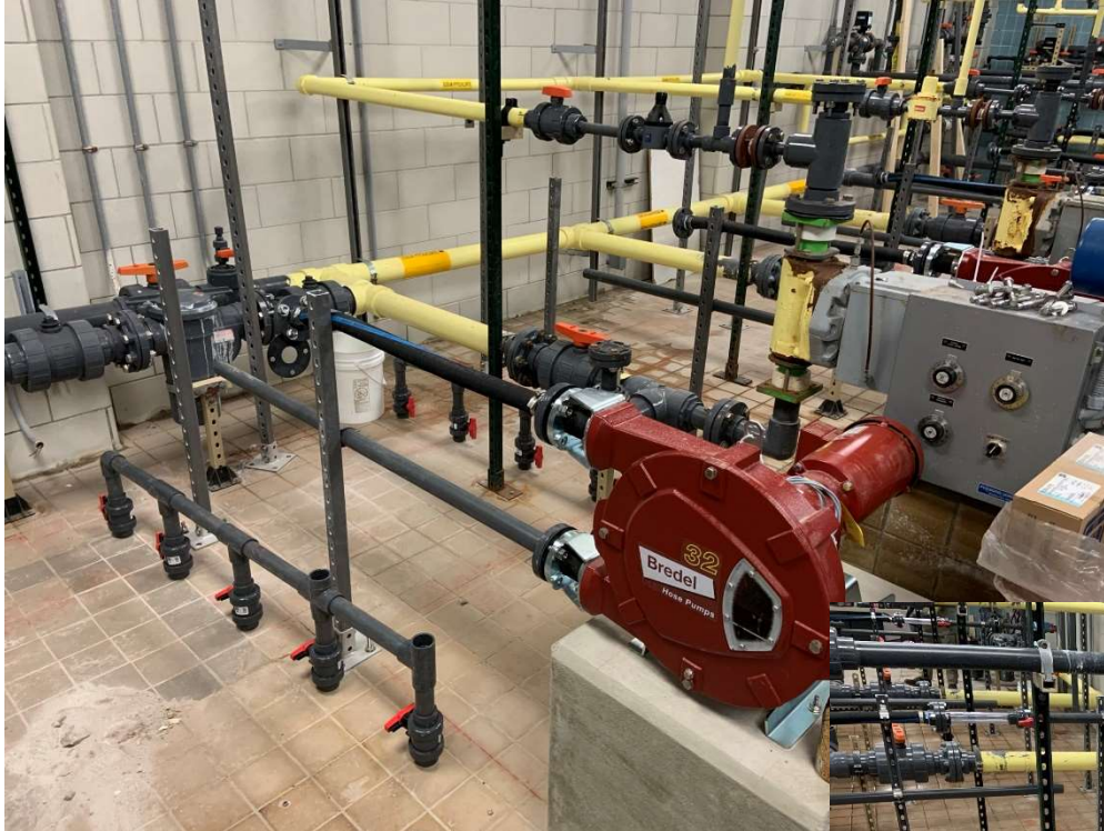
Figure 4 – New Pumps installed at Chapaton (new manifold staged on floor)
