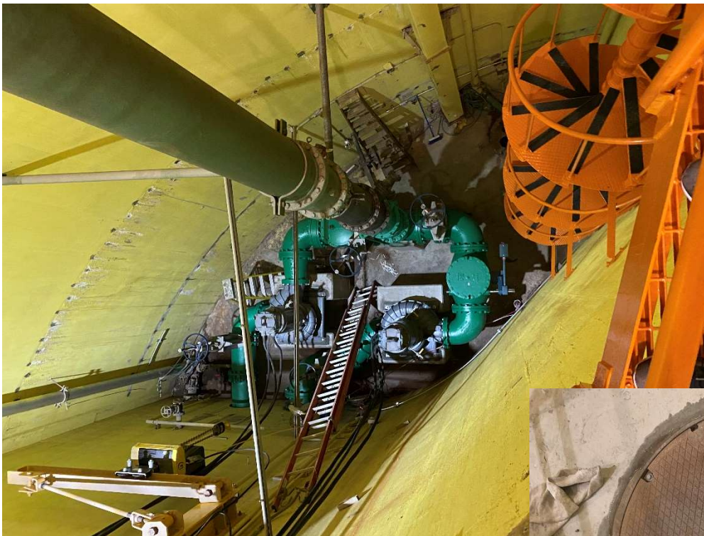
Figure 1 - Pumps installed and painted
