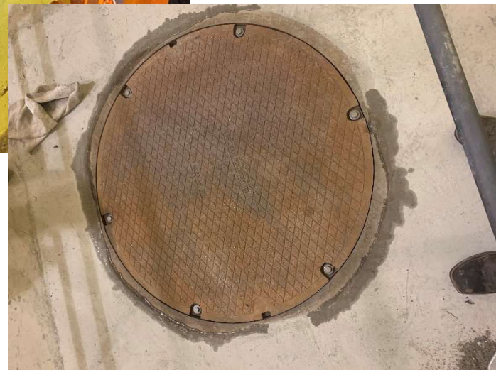
Figure 2 - New Manhole Cover
