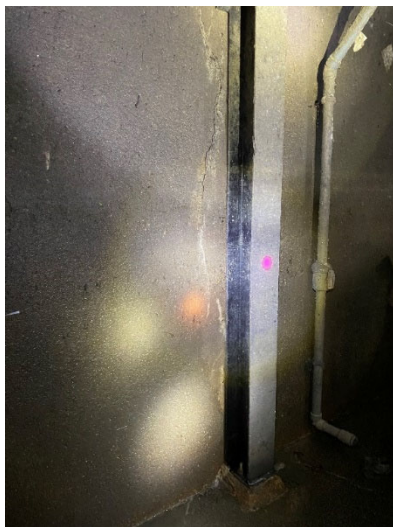
Figure 1 – Crack at Support Column / Joint
